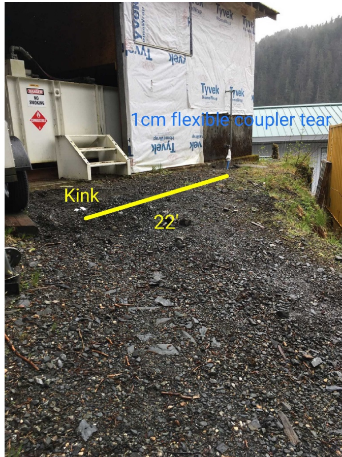
Figure 4. Workshop and generator shed area: Location of kink and leak.
