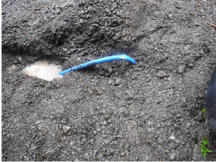
Figure 5. Workshop and generator shed area: Kinked fuel line.
