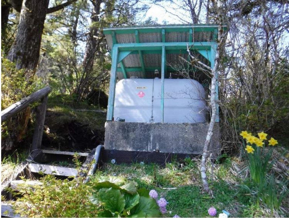
Figure 12. Storage tank at Pan Abode Cabin with history of spill
