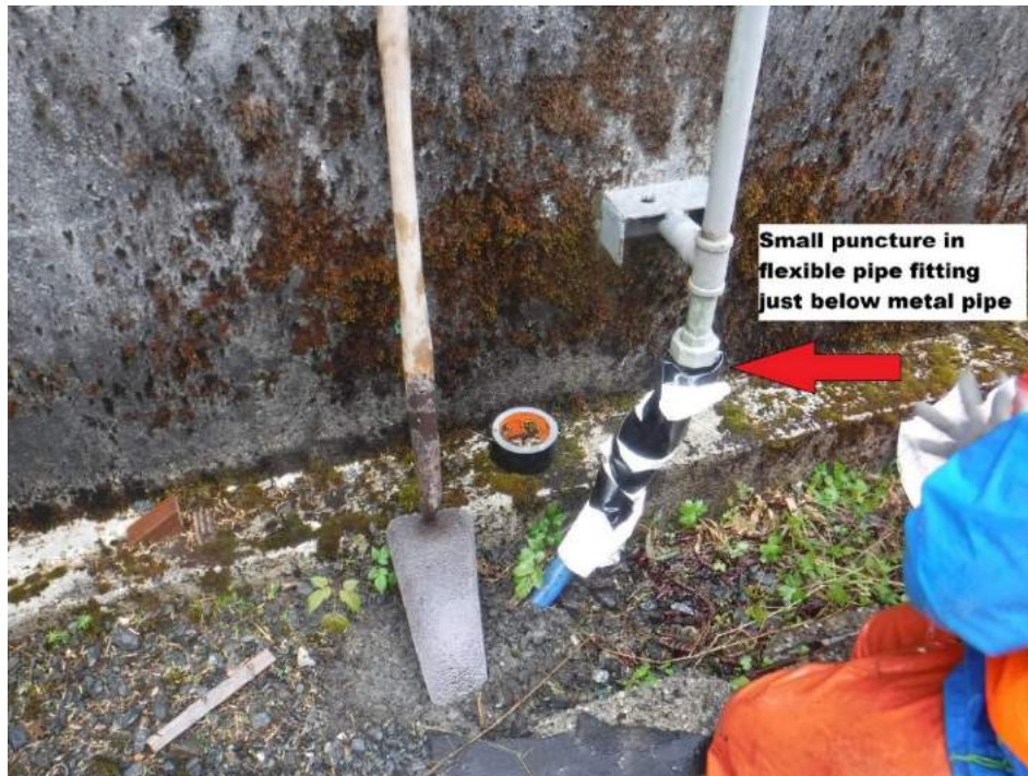
Figure 7. Workshop and generator shed area: Location of leak.
