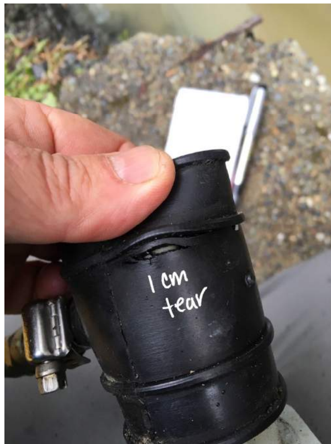
Figure 8. Workshop and generator shed area: Flex fitting leak.
