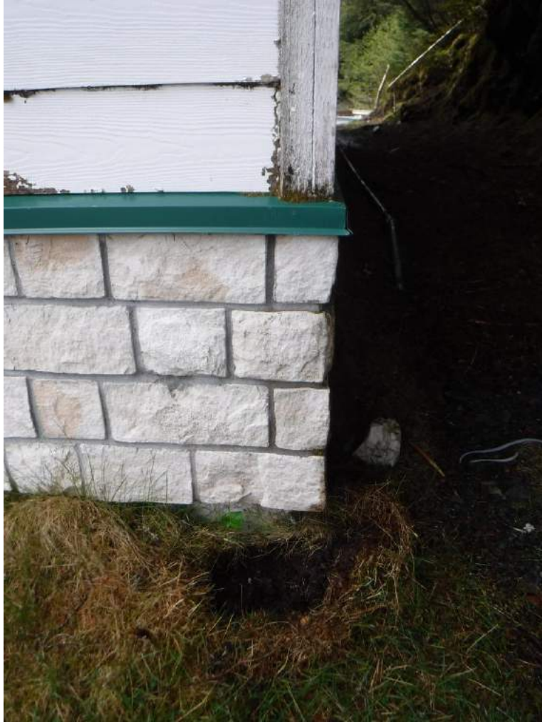
Figure 14. LBP and Treated Lumber soil sample along dripline of White House
