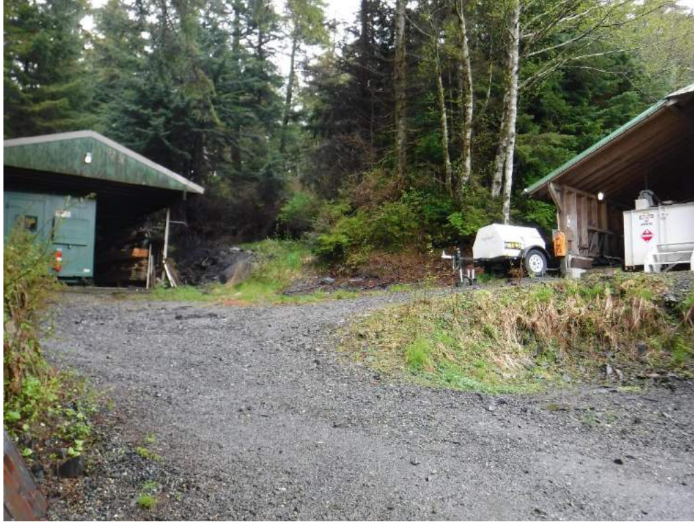
Figure 6. Generator Shed and Bulk Fuel Tanks
