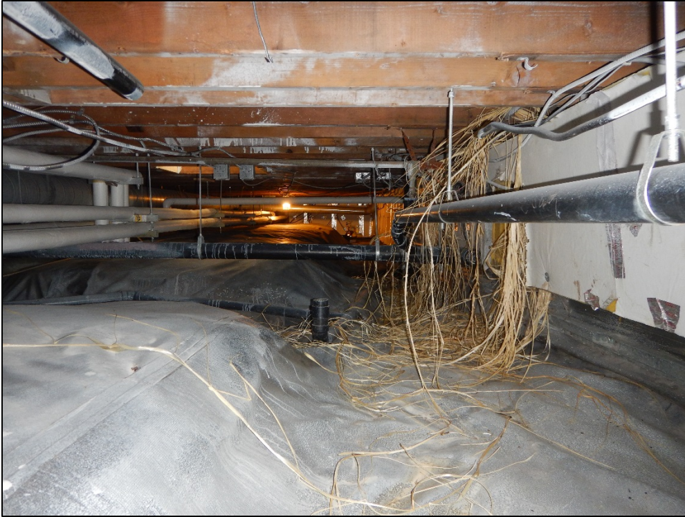
Photograph 11: Grass growing through foundation wall in crawlspace. Looking east.
