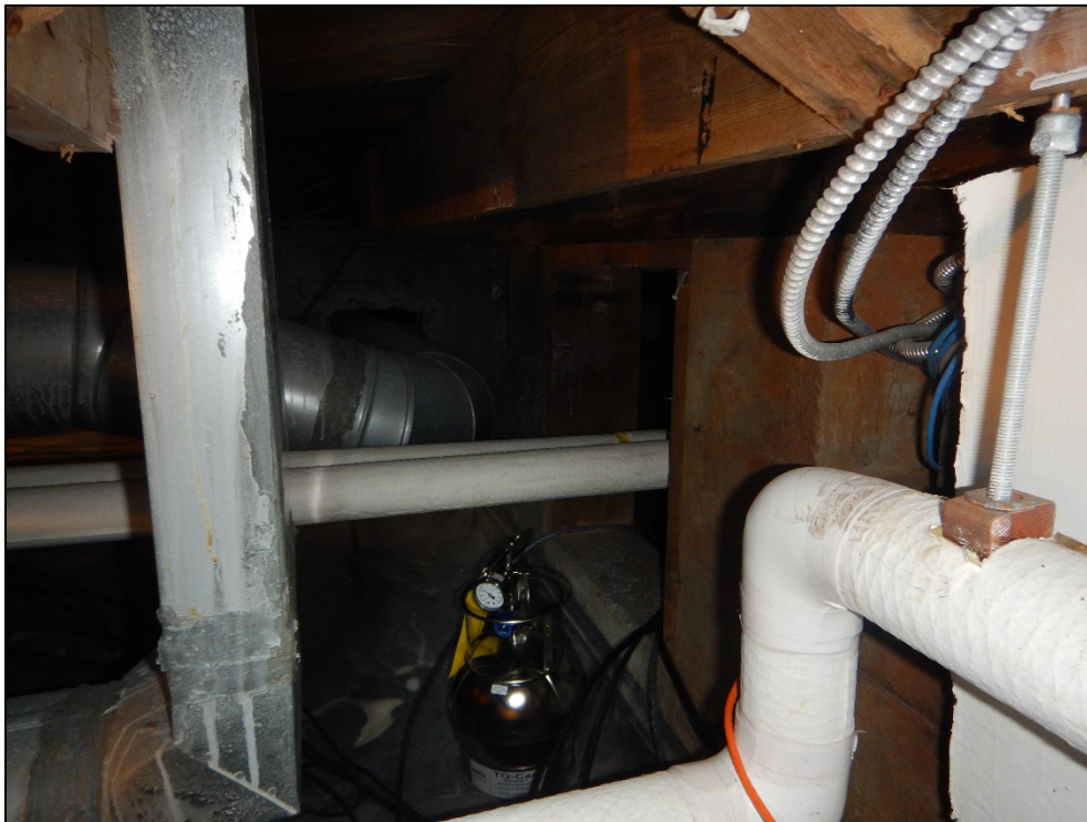
Photograph 12: VS2 sample location. Hole through wall to east is visible. Looking northeast.
