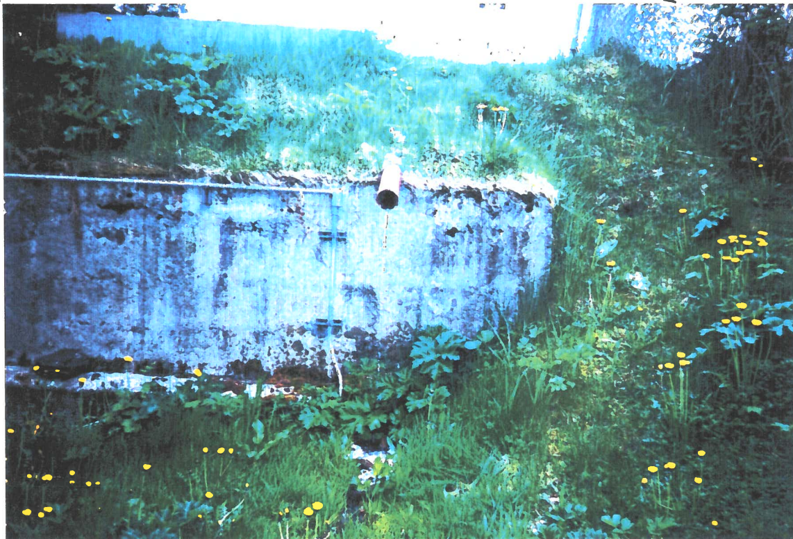
TTLR STORM/COLLECTION WATER DISCHARGE POINT
