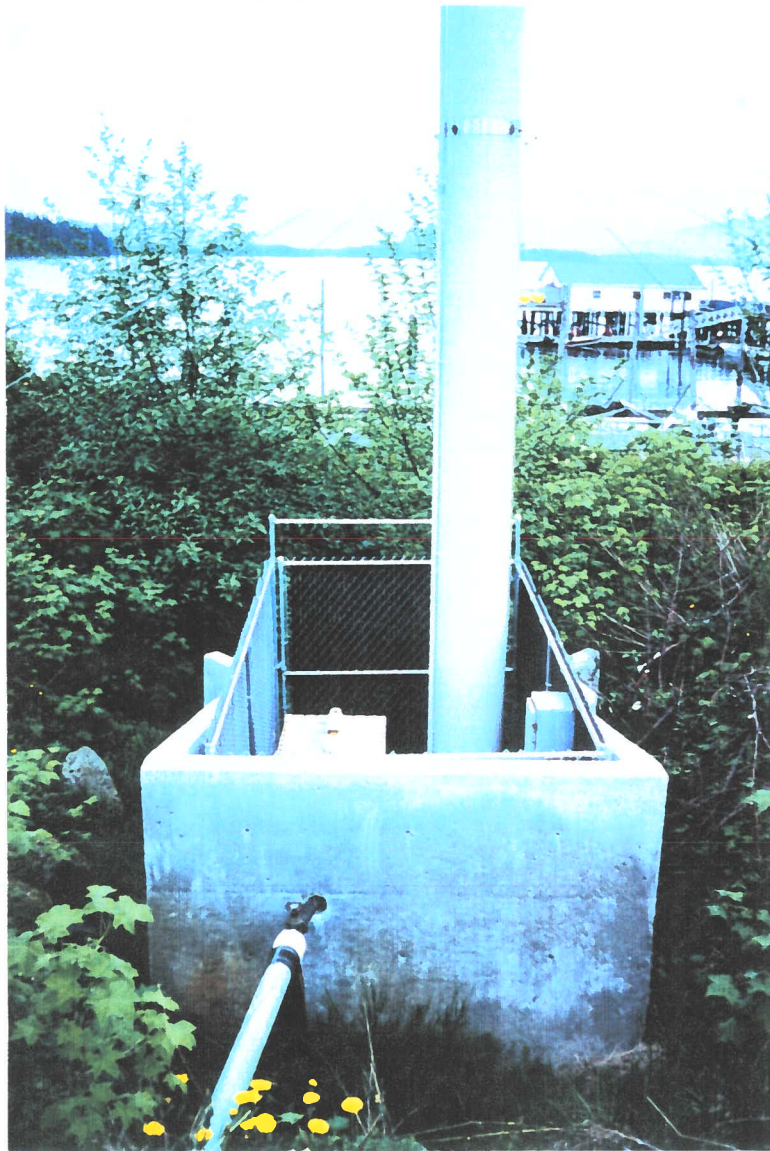
AIR STRIPPING TOWER
