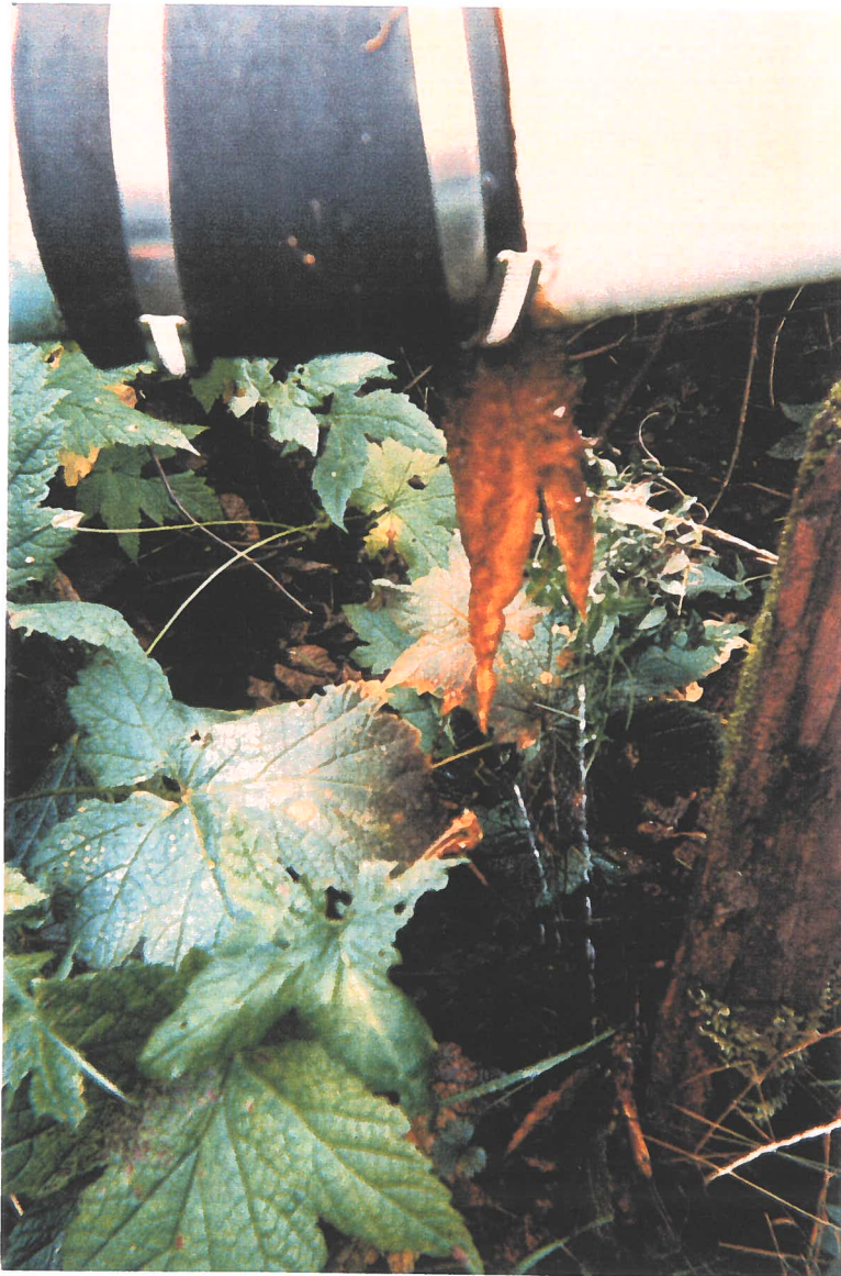
Photo 5. Close up of brown biomass growing under leak in air stripper piping. Note water dripping to ground.
