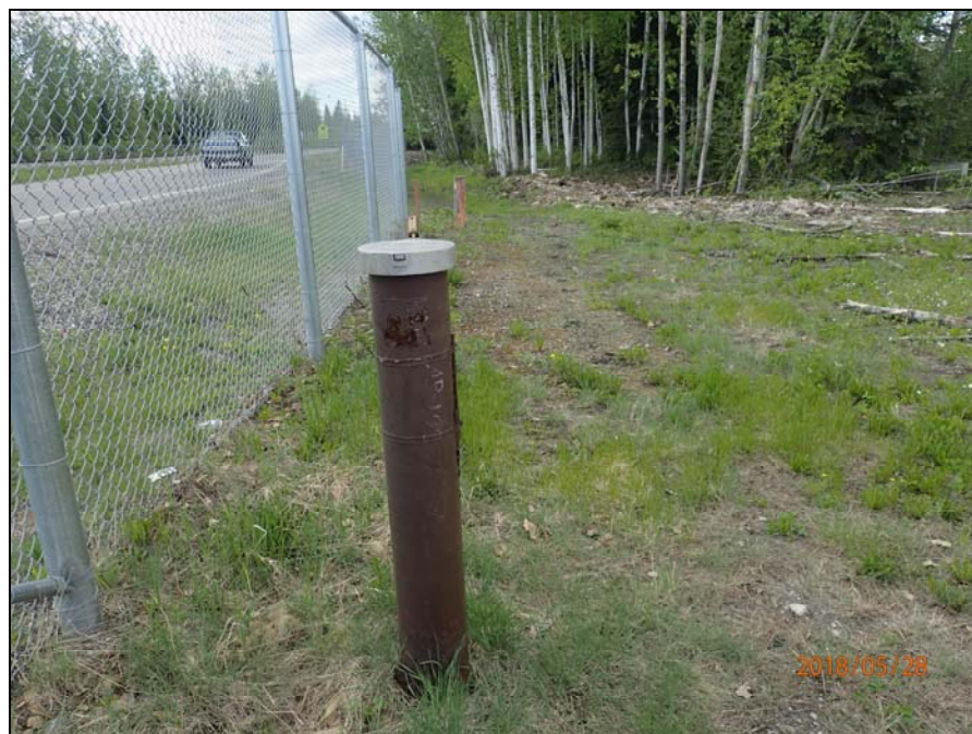
AP-10037MW closeup (view to the W)
