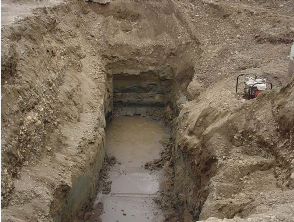
Photograph A2-1: Final excavation on 5/1/07 with groundwater and free-phase hydrocarbons prior to pumping
