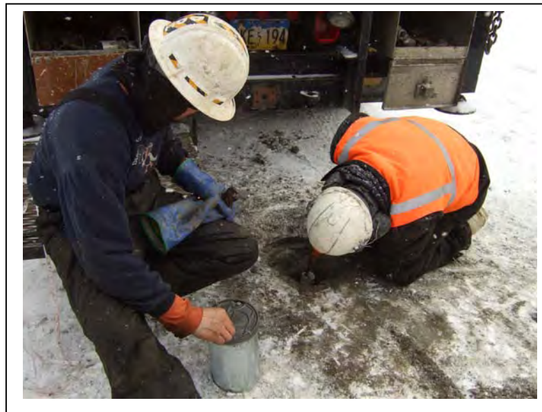
Photo 2: Monitoring Well B2MW was installed in Boring B2. In this view, the well casing is being trimmed down to allow installation of the flush-mount protective casing. (February 22, 2013)
