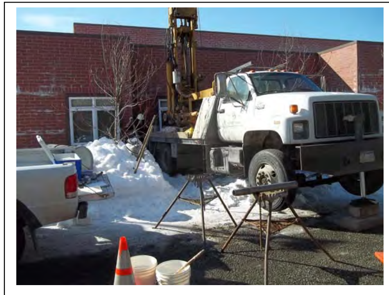
Photo 6: Boring B4 was advanced on the north side of Fire Station No. 4; looking south-southwest. (April 15, 2013)
