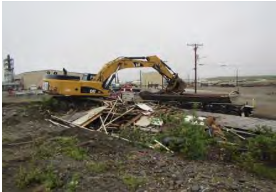
Photo No. 16 – 20 June 2016 Demolition material being loaded for transport to the landfill. Looking northeast.
