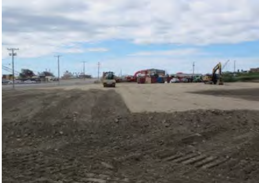
Photo No. 17 – 26 June 2016 Site preparation and compaction of cap footprint. Looking south.
