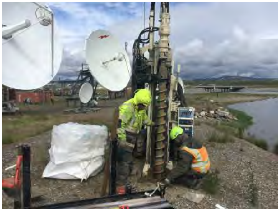
Photo No. 8 – 18 June 2016 Hollow-stem augers used during installation of W-36; well was relocated due to microwave dish shown in background. Looking north.
