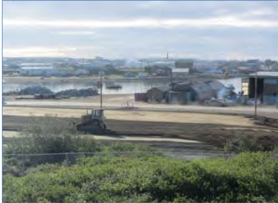
Photo No. 21 – 14 July 2016 Spreading and compaction of top layer of cap. Looking east.
