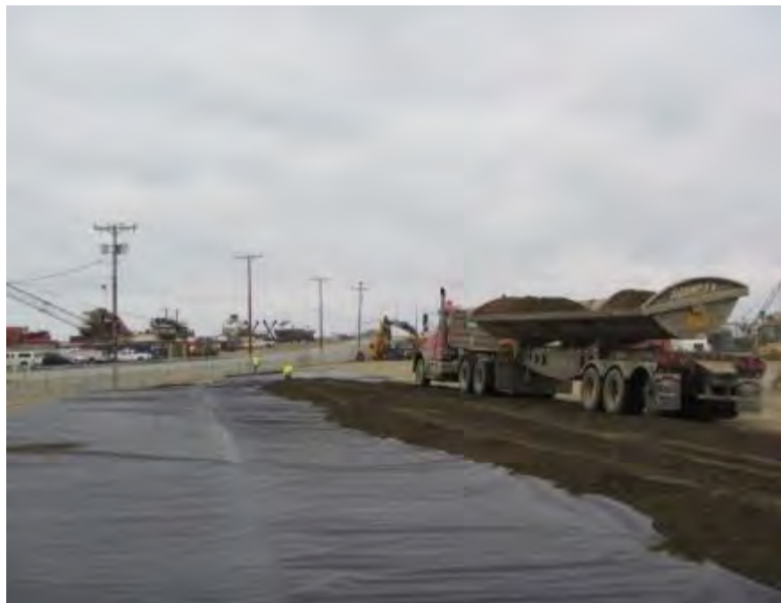
Photo No. 18 – 30 June 2016 Delivery of silty-sand base on top of geotextile liner. Looking south.
