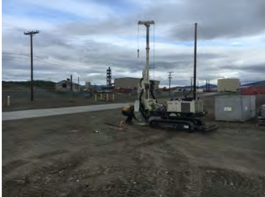
Photo No. 10 – 19 June 2016 Drilling step-out borings (B01 – B04) around W-17R. Looking north.
