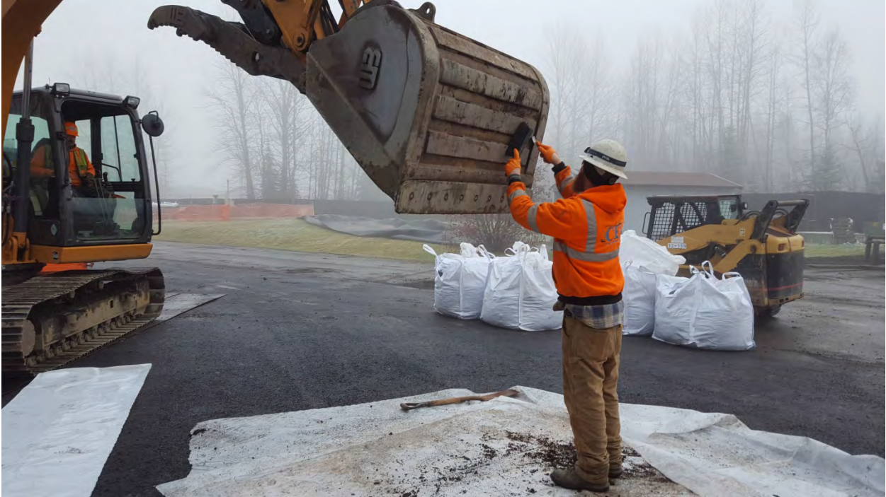
Photo 9: Dry decontamination of excavator bucket after excavating soil from AOC08-005. November 3, 2017 facing east.
