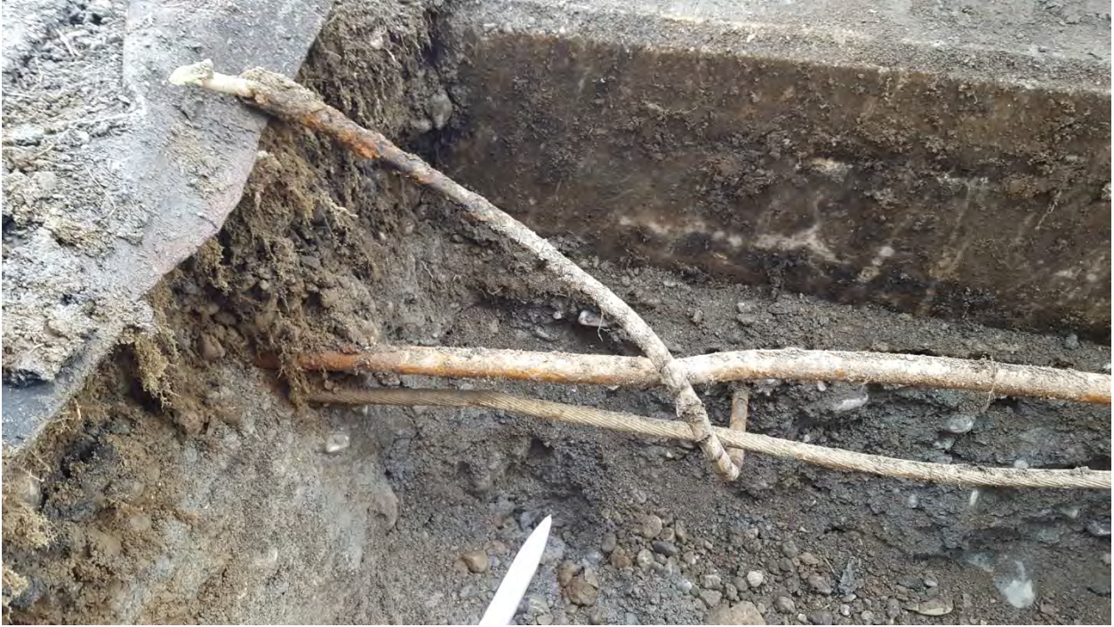
Photo 3: Cables encountered during excavation of AOC02-008. November 4, 2017 - facing east.
