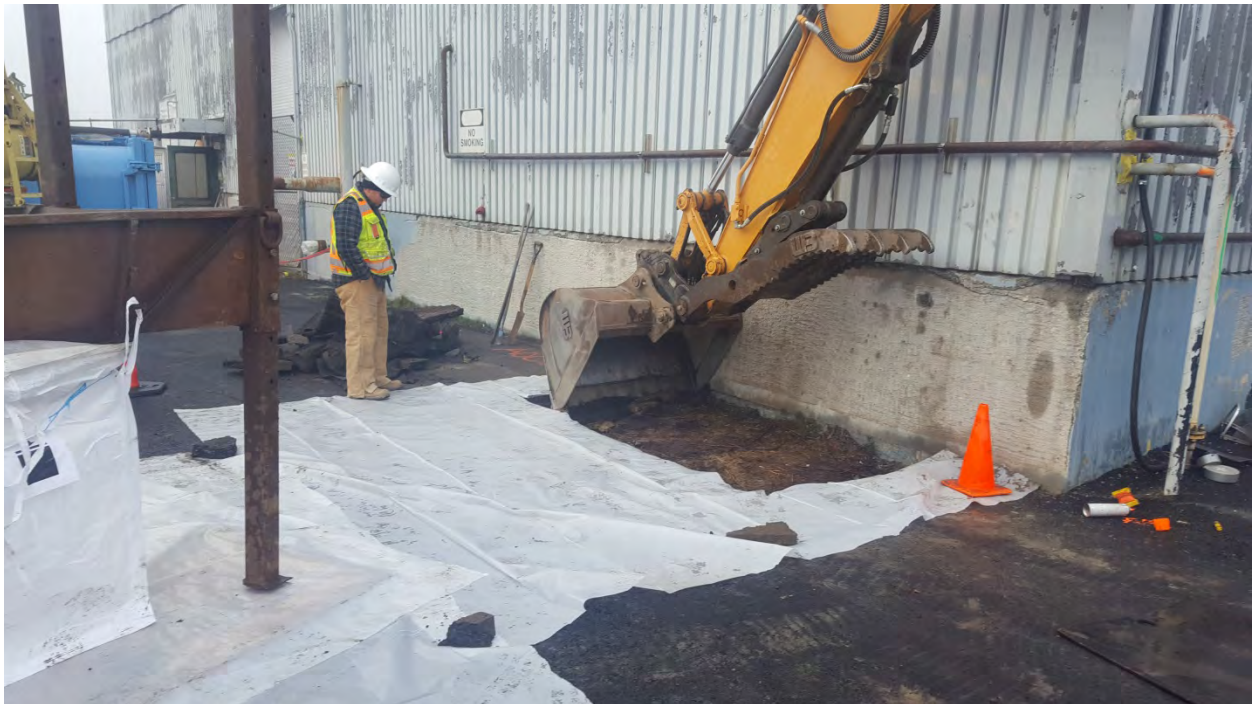
Photo 8: Excavation of AOC08-005. See soil hopper is on the left. November 3, 2017 - facing northwest.
