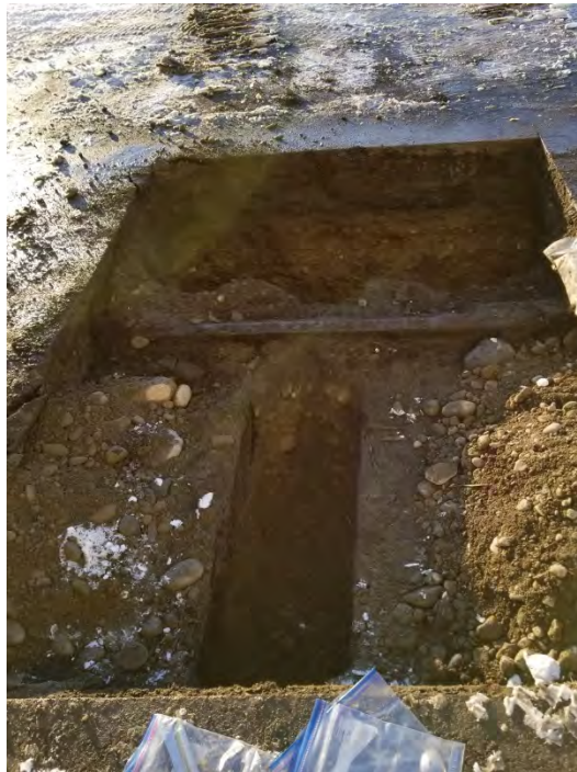
Photo 6: AOC07-002, showing full-depth excavation between 2 railroad ties in the foreground, and on the fare side of the rail. Coal is also visible in the far sidewall. November 6, 2017 - facing west.
