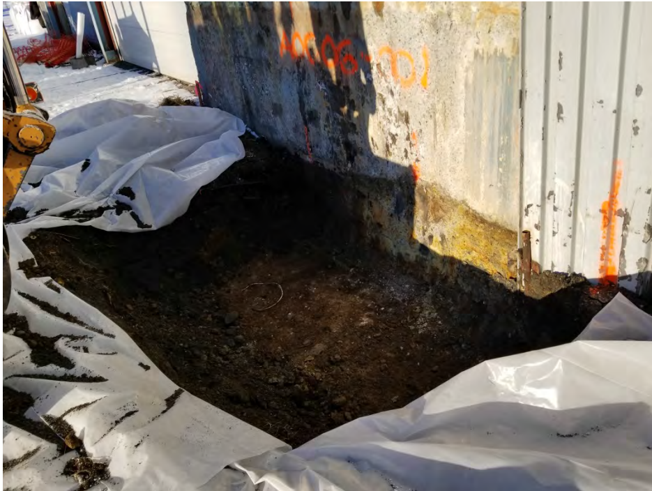
Photo 4: AOC06-001. Acid Vent location. November 6, 2017 - facing west.
