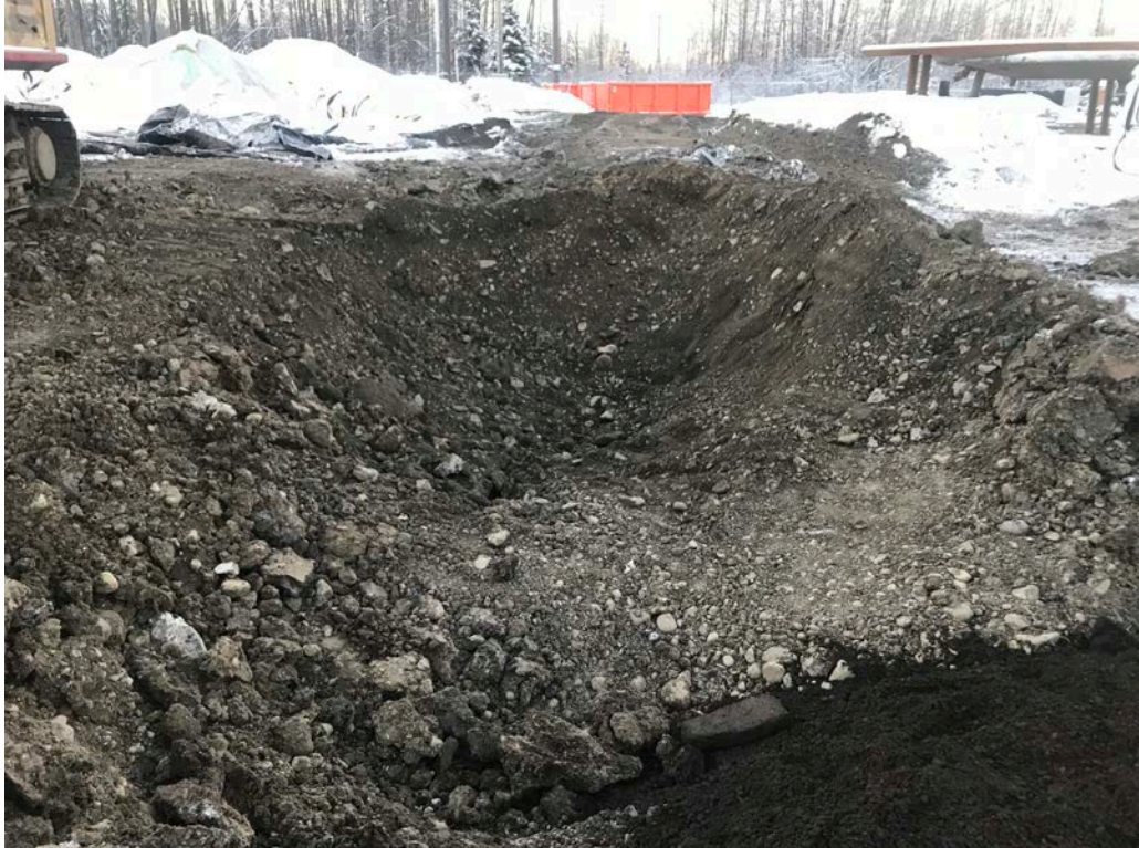
Photo 1: This photo shows the excavation under the former utilidor pump house, facing south. (October 31, 2018)
