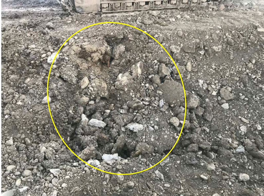
Photo 3: This photo shows the east sidewalls where non-native soil has started to be used as backfill. The non-native soil is shown in the circle. (October 31, 2018)
