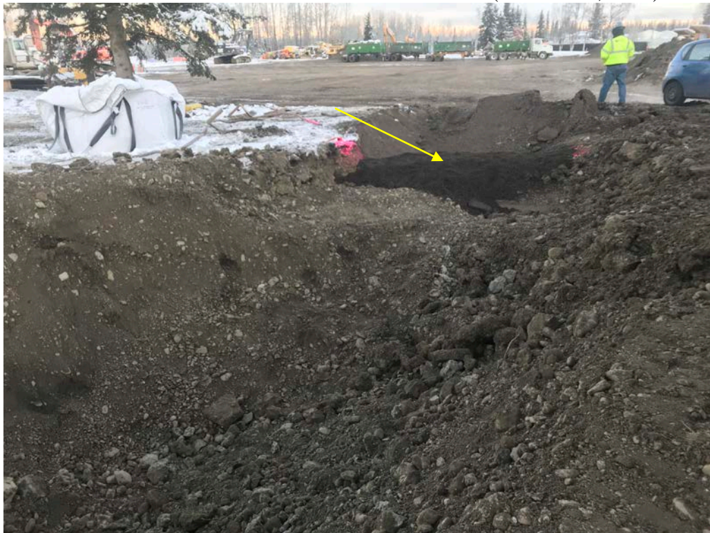
Photo 4: This photo shows the excavation, facing north, the utilidor excavation had been previously screened and backfilled. The arrow shows the soil that was backfilled on October 31, 2018. (October 31, 2018)
