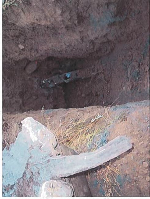
Photo 8. Debris and impacted soil encountered in Test Pit Six.
