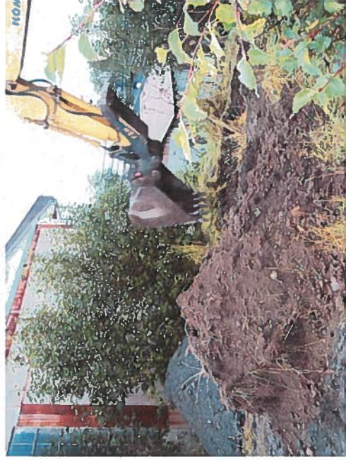
Photo 7. Breaking Ground at Test Pit Six located to the South of the Garage (Looking North)
