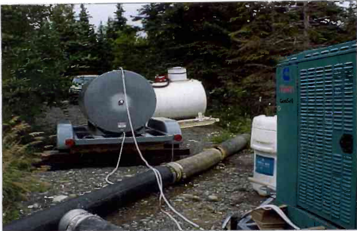
OUC: Eagle River Flats, View of Generator Set, Spill Kit, Diesel AST's and Large Water Pipe.
