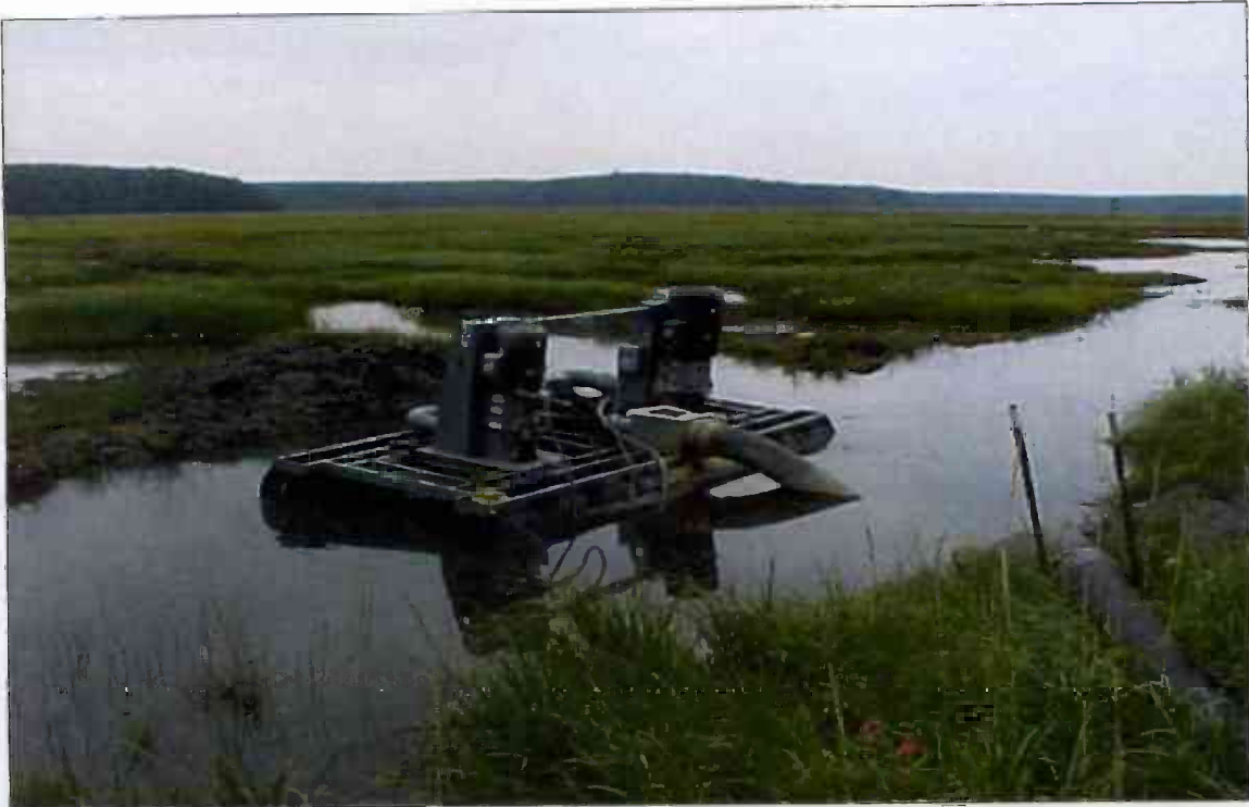
OUC: Eagle River Flats, View of Large Water Pumping System.
