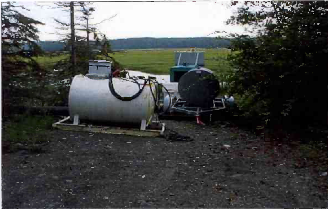
OUC: Eagle River Flats, Diesel AST's and Generator Set for Water Pumps.
