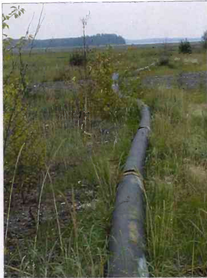
OUC: Eagle River Flats, Pipeline to Transport Water from Ponds to Knik Arm.
