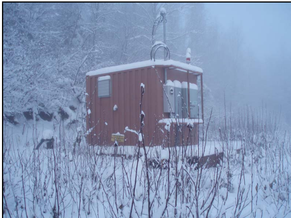
Photograph 2. Treatment system connex at OUB Poleline Road Disposal Area
