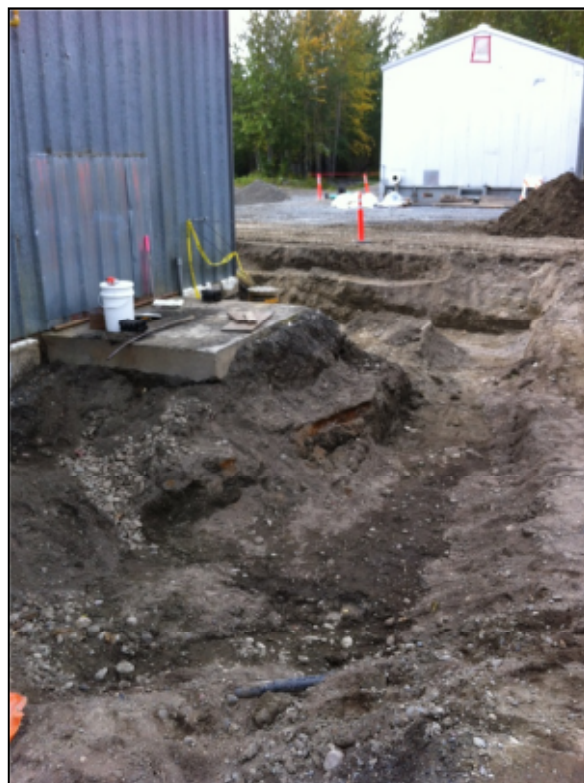
PHOTOGRAPH 2: VIEW OF THE EXCAVATION AREA AFTER PIPE WAS REMOVED, LOOKING WEST (SEPTEMBER 2012)
