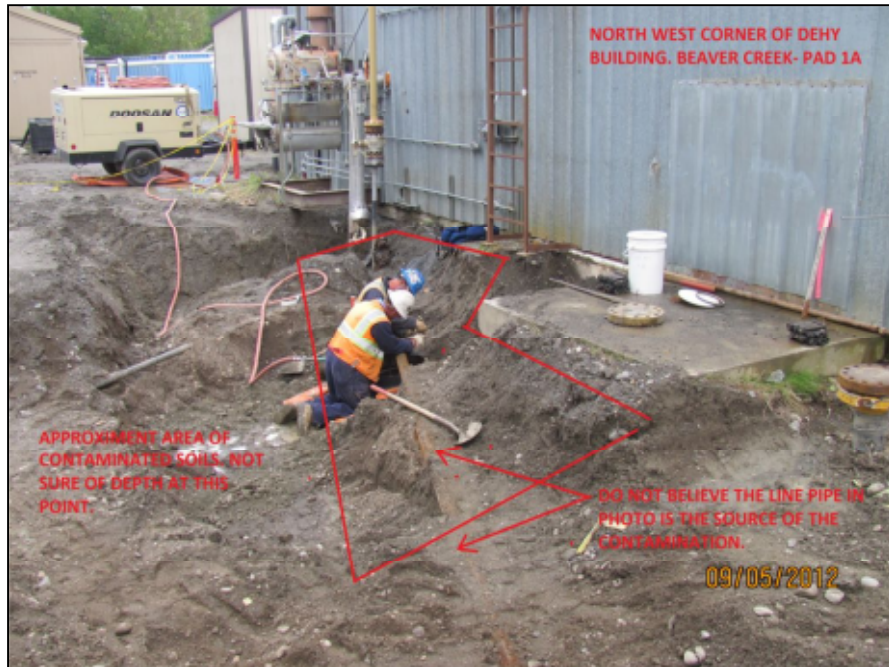
PHOTOGRAPH 1: VIEW OF THE EXCAVATION AREA, DEHYDRATION BUILDING, AND LOCATION OF PIPE BEFORE IT WAS REMOVED, LOOKING EAST/SOUTHEAST (SEPTEMBER 2012, COURTESY OF CH2MHIL)
