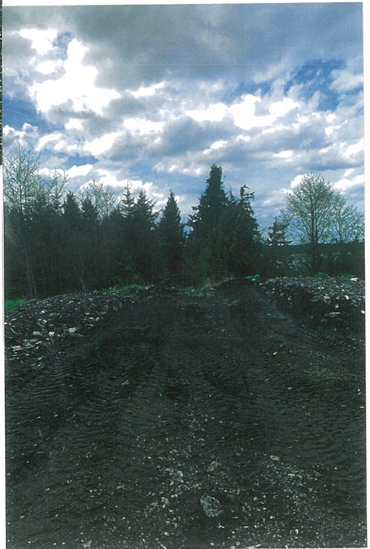
Photo #2: 5/4/20 view looking SW between Biocells #3 & #4, where its adjacent rocked containment berms had been removed and used as fill for the PL-33 excavation.
