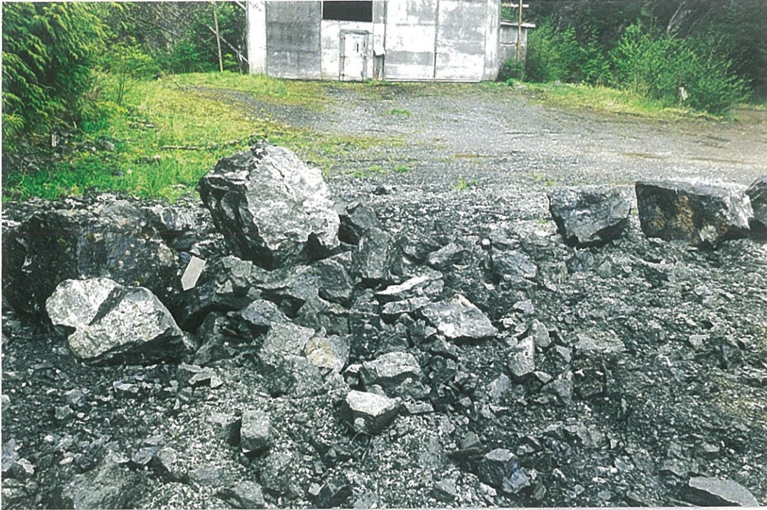
Photo #15: 5/6/20 view looking at the area in front of the Phoenix Logging shop, where the groundwater well pipe (arrow) had just been removed and the area backfilled.
