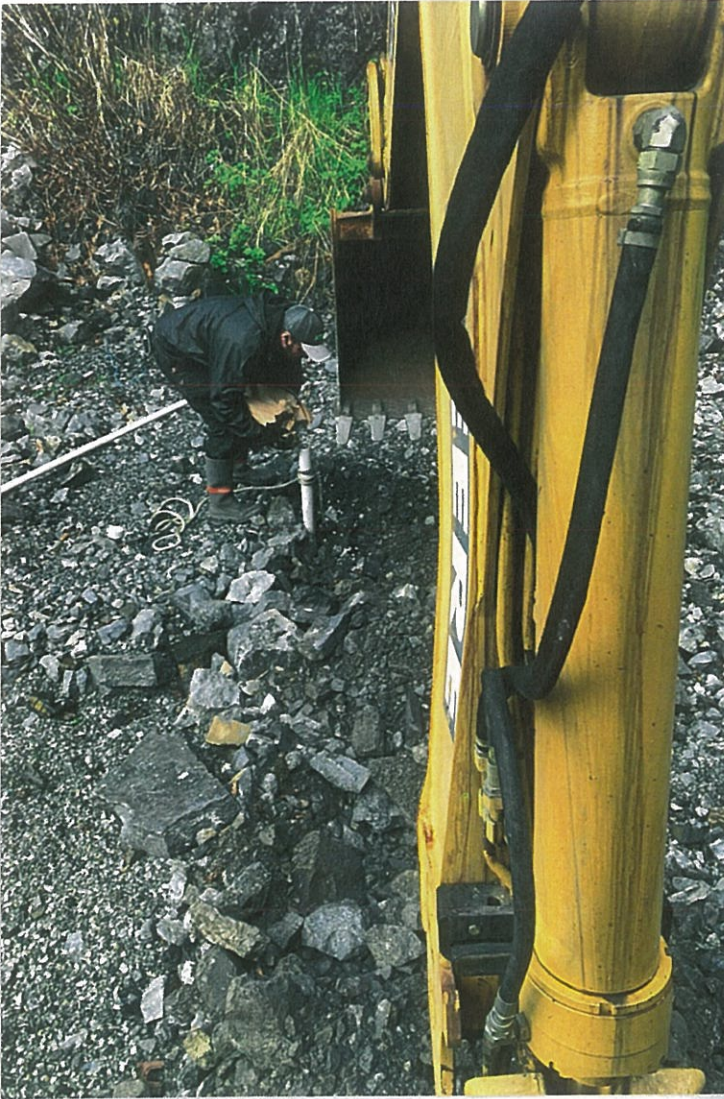
Photo #13: 5/6/20 view of the groundwater well pipe stem in the back of the Phoenix Logging shop, as bentonite chips were being poured down the pipe. Once the chips were rammed out the bottom of the pipe, the backhoe pulled the pipe about 1'-1.5' out of the ground, and additional bentonite was poured into the pipe (see photo below).
