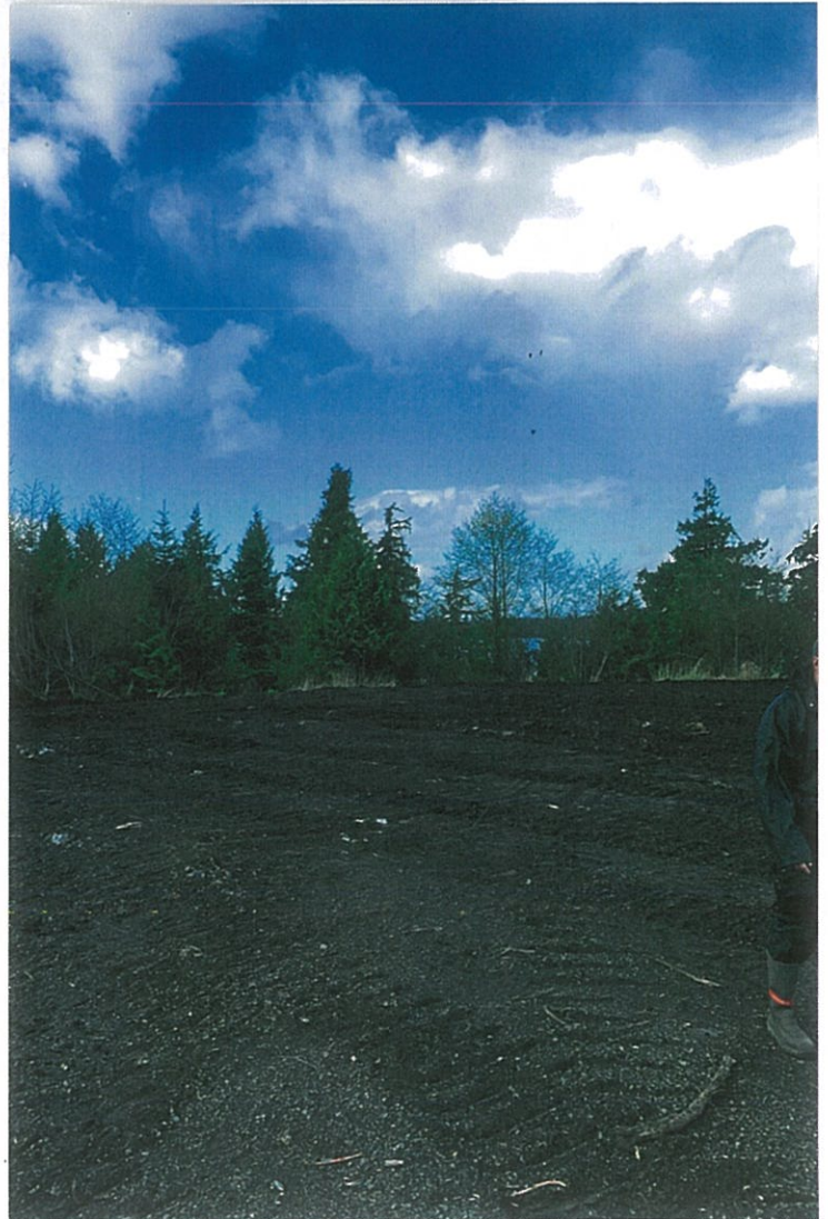
Photo #8: Closer 5/5/20 view looking SW across the upper end of the Biocell #1's soils, after being bladed and smoothed with the D9 cat to a 5"-6" thickness throughout.
