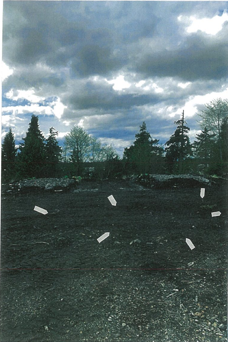
Photo #3: 5/4/20 view looking SW between Biocells #2-#3, showing the removed containment berms without affecting the biocell soils. Arrows show the approximate perimeter of the backfilled PL-33 excavation (see also next photo).
