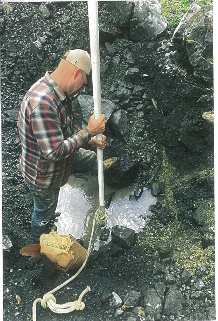
Photo #12: 5/6/20 view of more bentonite chips being poured down the groundwater pipe stem, after which the bentonite was rammed down the pipe and the backhoe pulled the pipe about 1'-1.5' out of the ground. More bentonite chips then were added, rammed down the pipe and then the backhoe raised the pipe an additional 6". This process was repeated until the pipe was completely removed from the ground.
