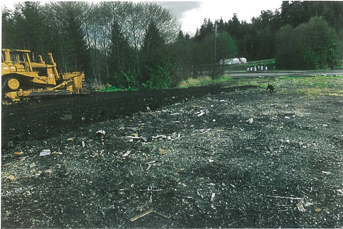
Photo #7: 5/5/20 view looking NE across the end of the Biocell #1 soils, as being spread to a 5"-6" thickness and a 180'-190' length.
