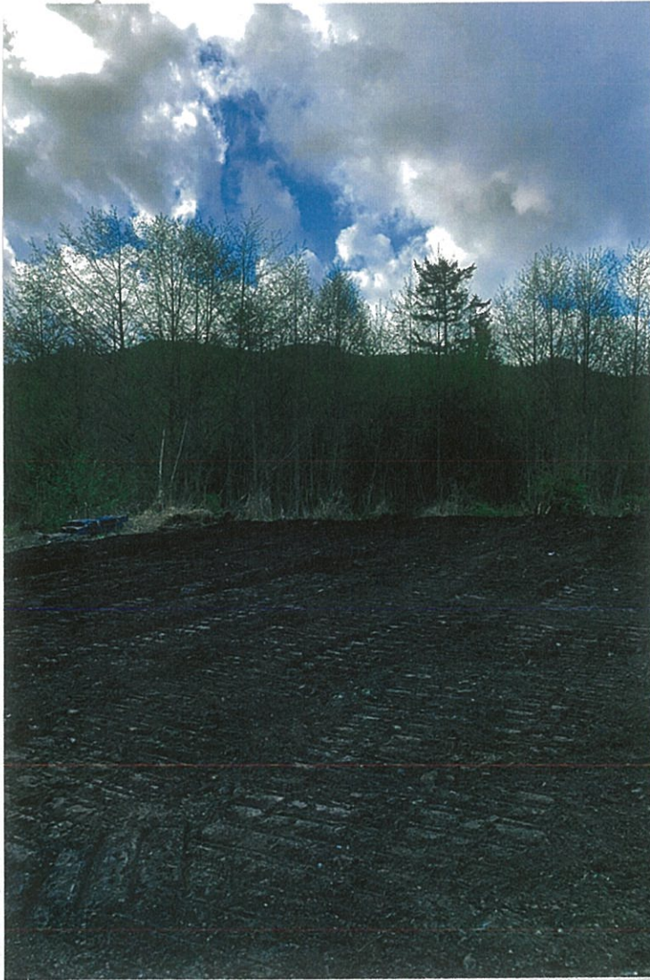
Photo #9: 5/5/20 view looking SSW across the far end of Biocell #4, after its soils had been spread to a 5"-6" thickness and contoured by the D9 tracks.
