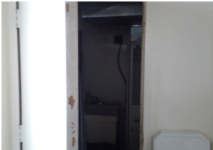
Photo 10. Kasaan Library furnace room
