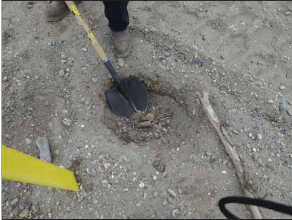
PHOTOGRAPH 7: MW-10 - BURIED 12-12 INCHES ON NEWLY PLACED GRAVEL PAD
