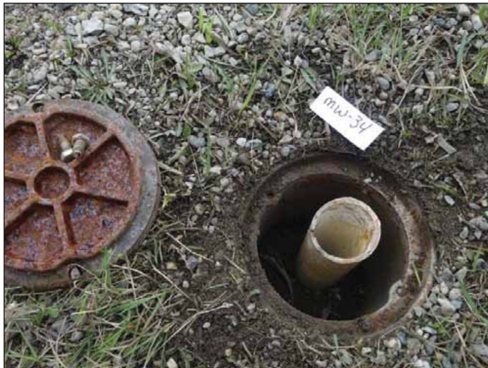
PHOTOGRAPH 18: MW-34 MODERATE CONDITION - CASING IS JACKED AND NO LONGER ABLE TO PLACE WELL CAP UNDER MONUMENT LID.
