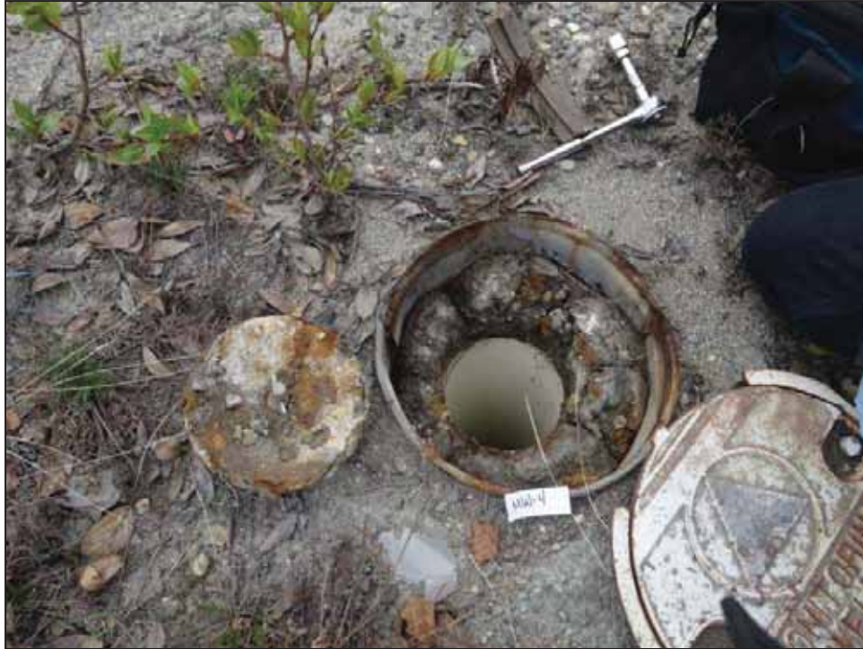
PHOTOGRAPH 3: MW-4 - POOR CONDITION, MONUMENT LID DOES NOT ATTACH AND BENTONITE SMEARED AROUND TOP OF CASING
