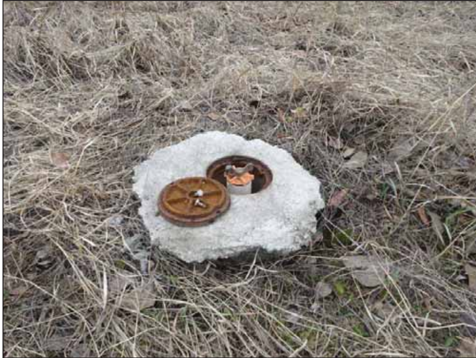
PHOTOGRAPH 19: MW-35 - MODERATE CONDITION - EVIDENCE OF FROST JACKING, CONCRETE IS NO LONGER BURIED.
