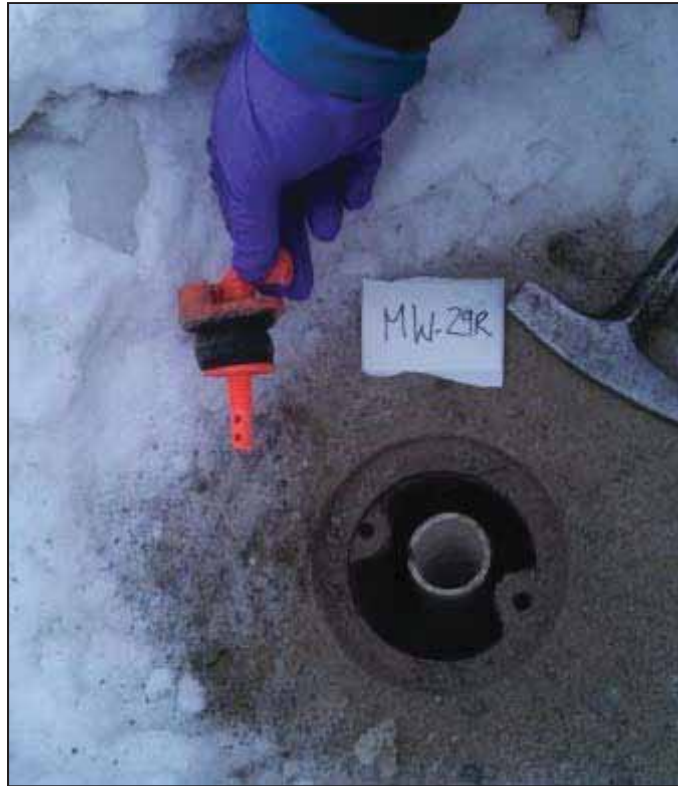
PHOTOGRAPH 15: MW-29R MODERATE CONDITION - CASING IS ALMOST TOUCHING MONUMENT LID - WELL REMOVED APRIL 2014
