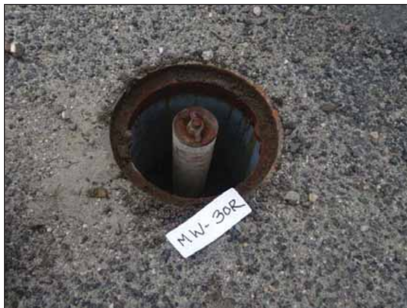
PHOTOGRAPH 16: MW-30R - MODERATE CONDITION - BLOCKAGE IN NOV. 2013 AND MINOR FROST JACKING
