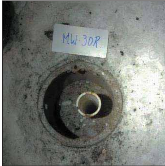
PHOTOGRAPH 17: MW-30R - MODERATE CONDITION - BLOCKAGE IN NOV. 2013 AND MINOR FROST JACKING
