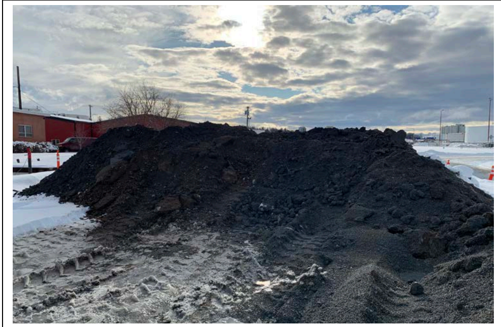
Photo 3: Looking south at the temporary soil stockpile, prior to transport to ASR. (February 20, 2020)
