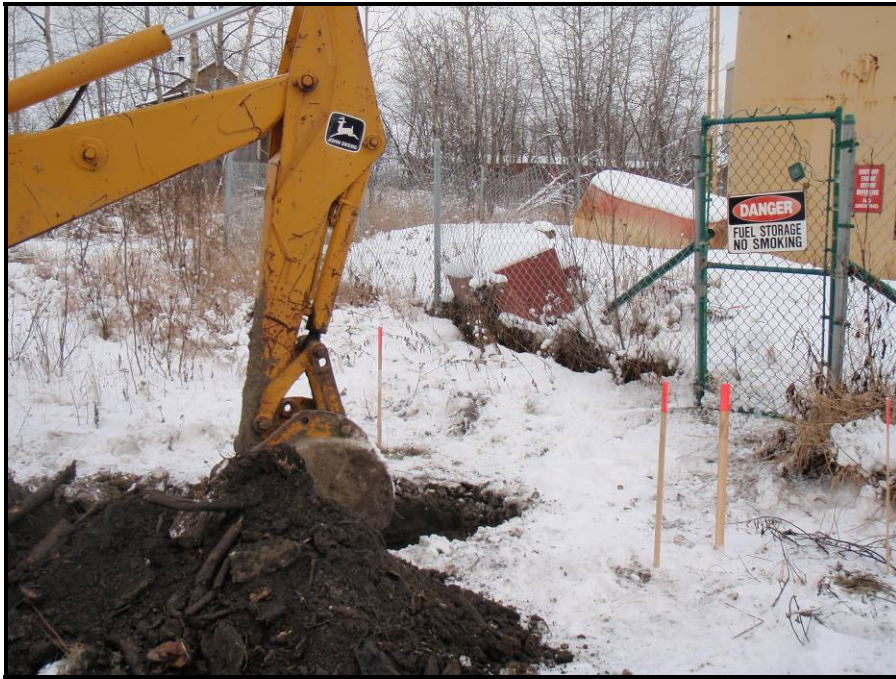
Photograph 9: Advancing Test Pit 1 in the old dispenser area; wood debris is visible in the soil pile in the bottom left corner of this photograph.
