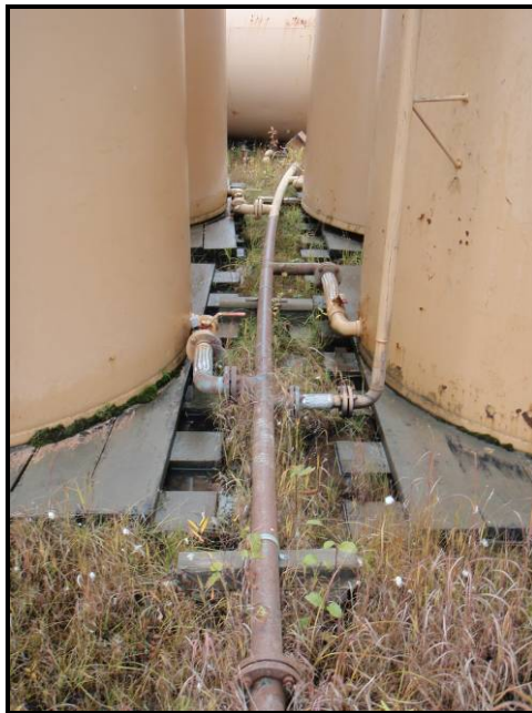
Photograph 2: Above ground piping within the diked area; all threaded piping was reportedly replaced with welded piping approximately eight years ago.
