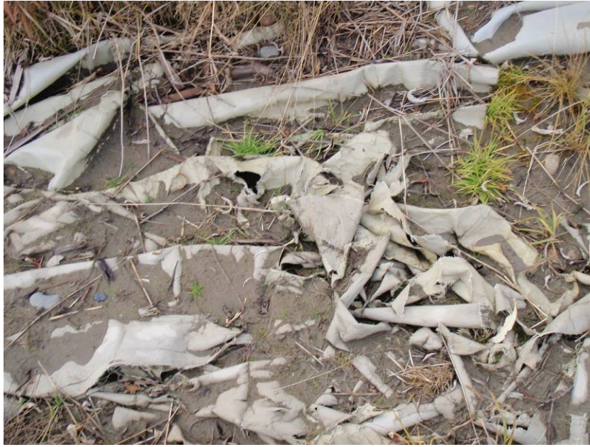
Liner damage at Old Corporation Tank Farm
