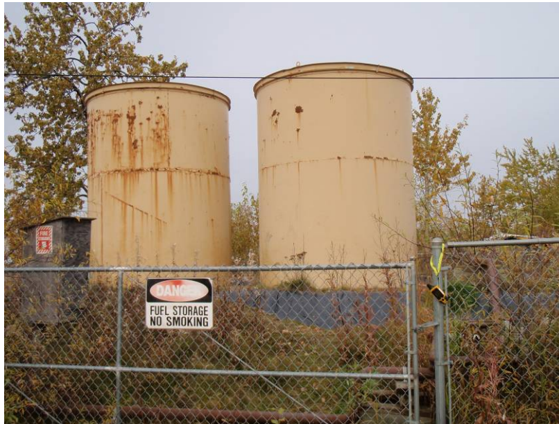
Old Elementary School Tank Farm
