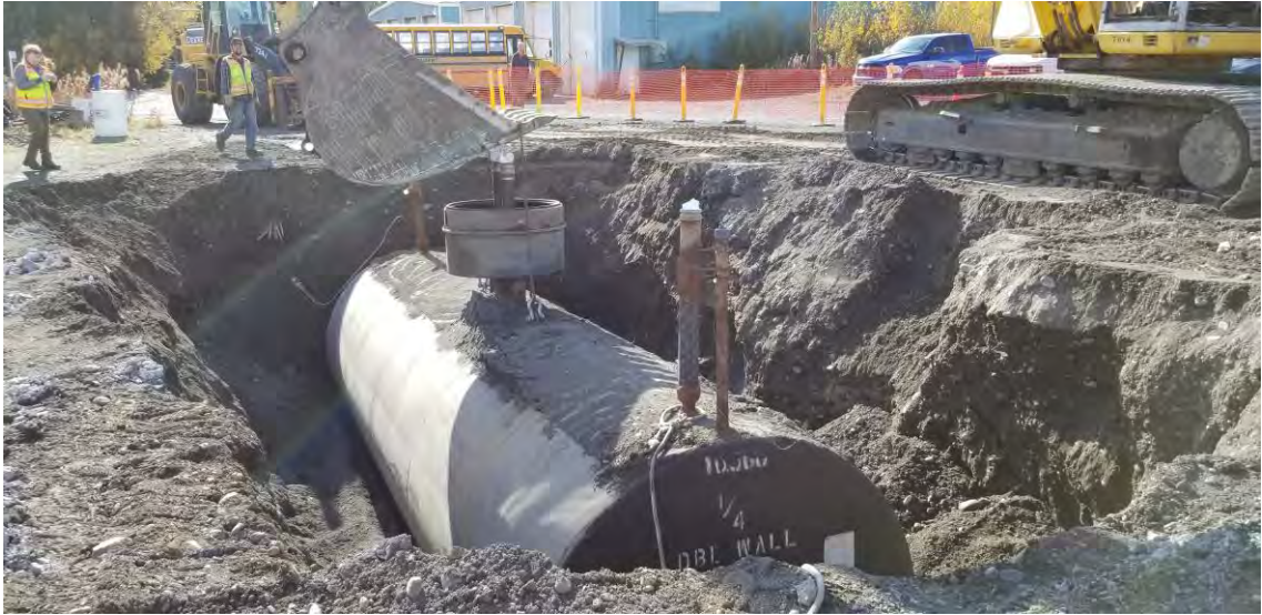
Photo 5: September 17, 2019, looking south - This photo shows the UST at the time of removal from the ground.
