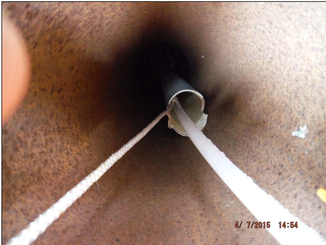
View of broken PVC riser at AP-5588
