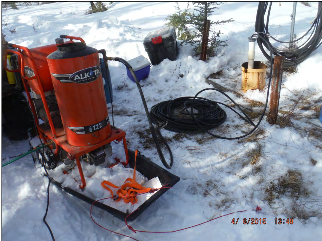
Thawing well AP-6532 with hot water due to failed dedicated heat trace.
