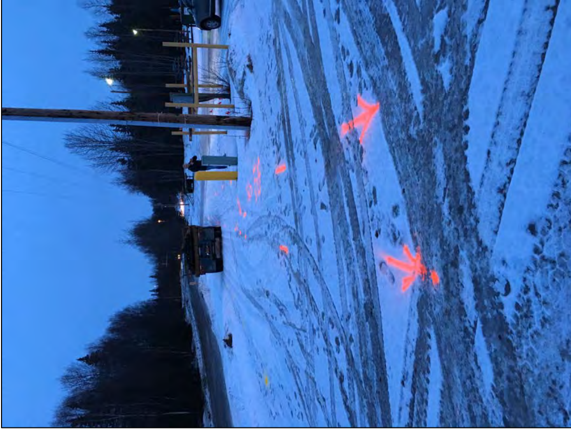
Photo: 1 Time: 1804 Date: 2/14/2016 Direction: West Subject: Utility locates completed at proposed SB-19/MW-09
