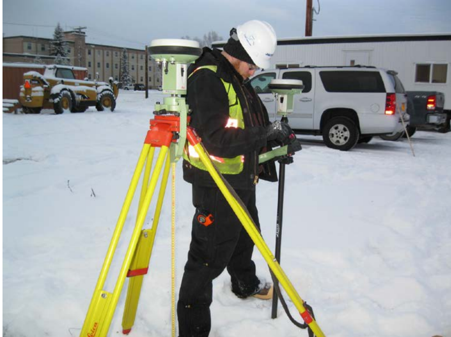
Photo No. 7 – 14 November 2012 Establishing survey control adjacent to Garrison Slough DU-7-1. View facing southwest.
