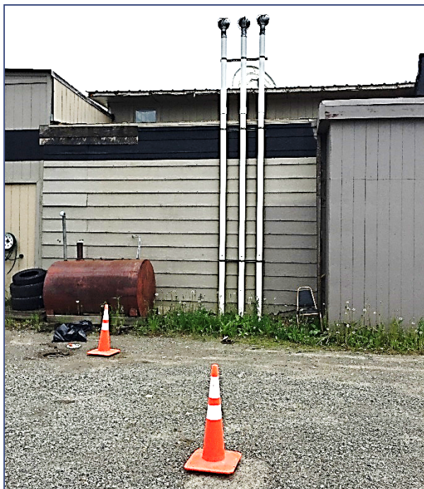
Exhibit 2-1: Wind-driven turbine ventilators mounted on the top of the passive remediation system on the north side of the building.
