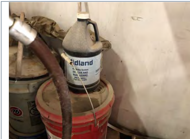
Photo 57: Air Brake System Inside the Shop Garage
