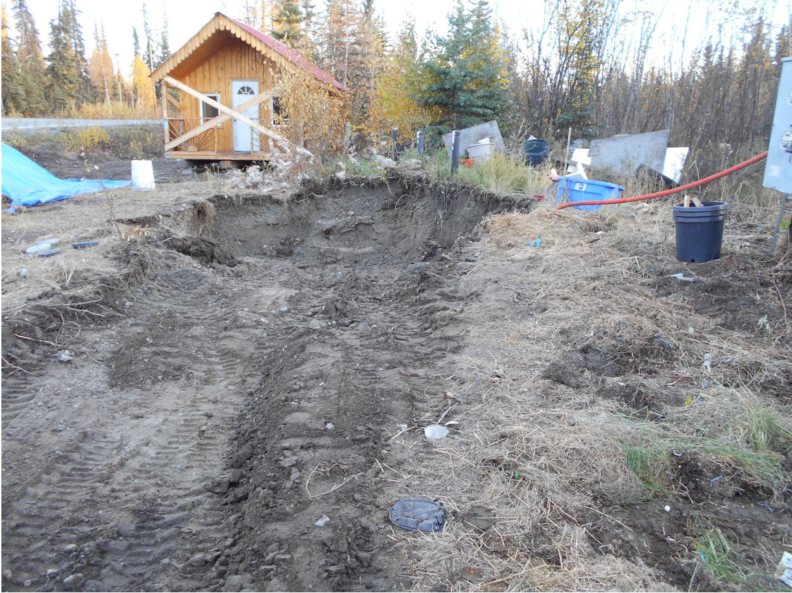
Figure 7. Looking east on September 27, 2013 at the former cabin and AST site after hydrocarbon-contaminated soils were removed and temporarily stockpiled under the blue tarp to the left in the photo
