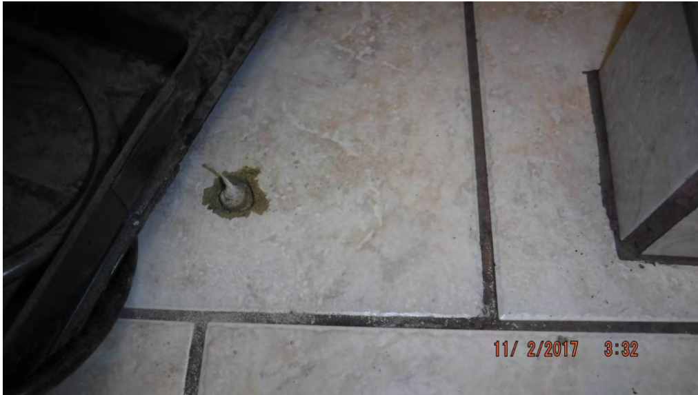
Photo 13: Sub-slab sampling port SS-03 installed inside the Buffalo Service Station storefront. (November 2, 2017)
