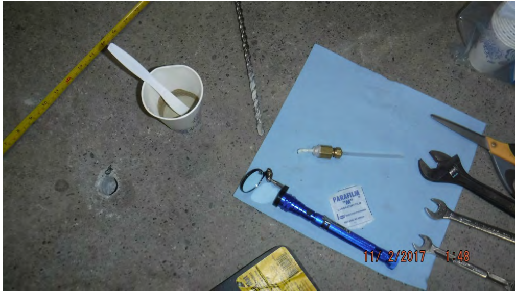
Photo 11: Preparing to install a sub-slab sampling port in the service station garage. (November 2, 2017)
