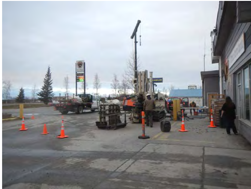
Photo 1: Setting up the drill rig in front of the Buffalo Service Center at boring location IT-B10 . (October 15, 2017)
