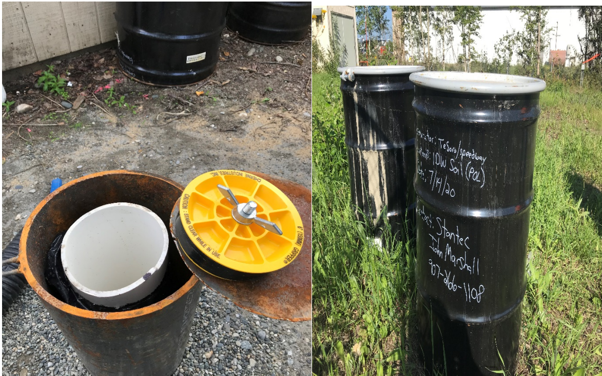
Completed WRW 2020 Well inside 10" Dia Steel Pipe 2 Drums of Soil Cuttings stored on-site for NRC Pickup
