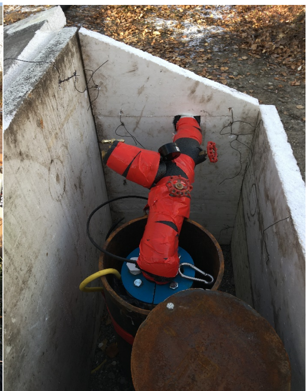
Insulated "DogHouse" over WRW 2020 Well Head
