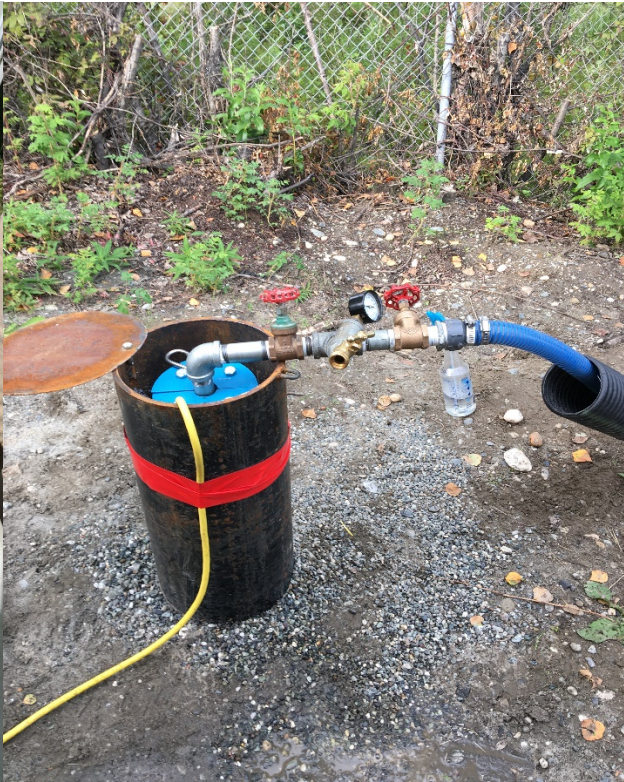
Flow Control Devices at well head on WRW 2020 Well
