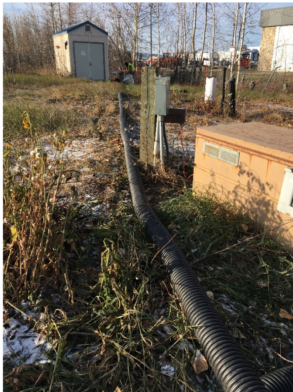
Water Line Discharge from WRW 2020 to Aeration Tank
