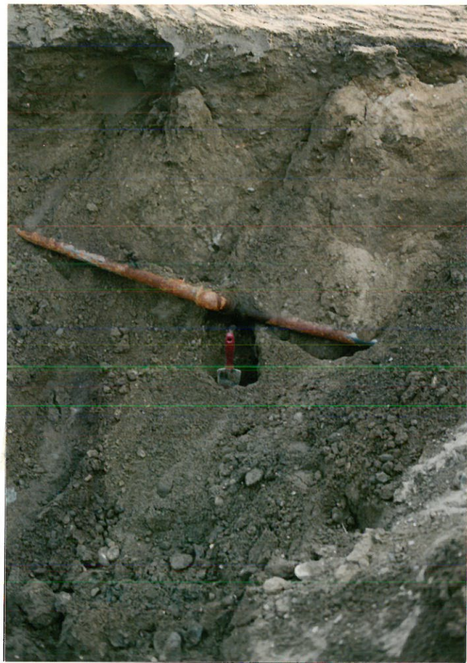
Photo #3: Product Piping Sample Location
