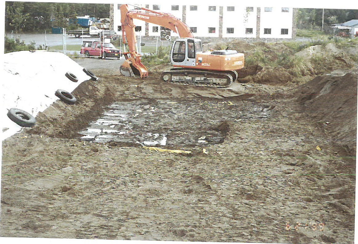
View to east. After stockpile liner removed and contaminated soil cleaned off heavy yellow liner under east end of stockpile.
