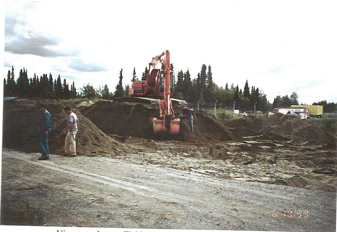
View southeast. Field screening soil in 600-700 cubic yard stockpile and placing in contaminated pile (on left) or clean pile (on right).
