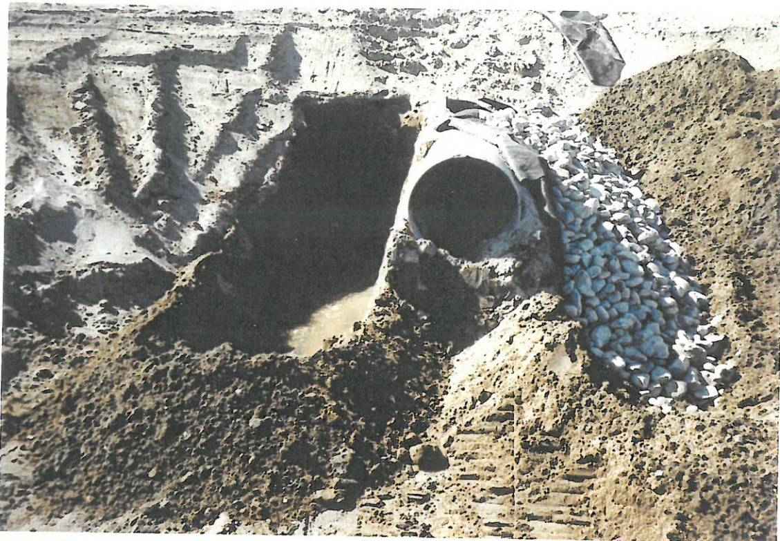
1) View to the West. Excavating around culvert. Note groundwater at the left side of culvert.
