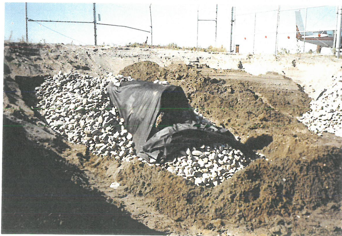
2) View to the Northwest. After drain rock and filter fabric were placed.
