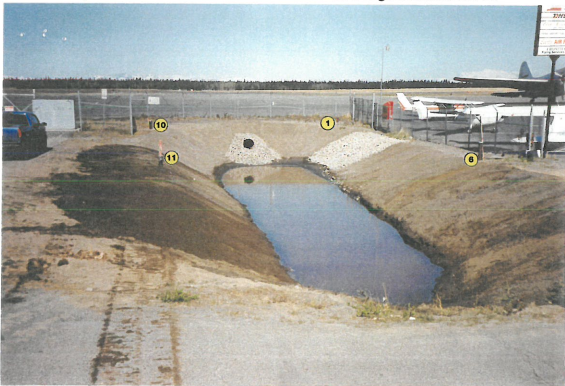
6) View to the West after excavation completed, before hydroseeding and fencing installed. Note location of existing MW-1 & 6 and new MW-10 & 11.
