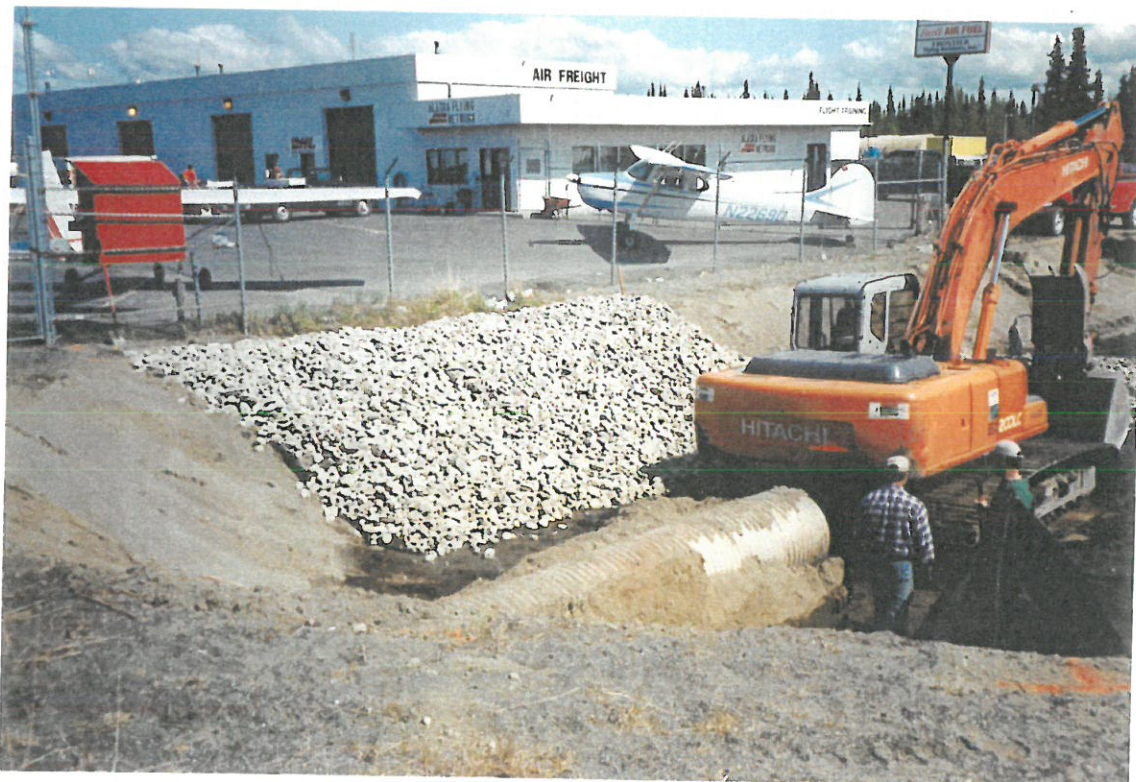
4) View to the Northeast. Placing filter fabric around culvert before placing drain rock.
