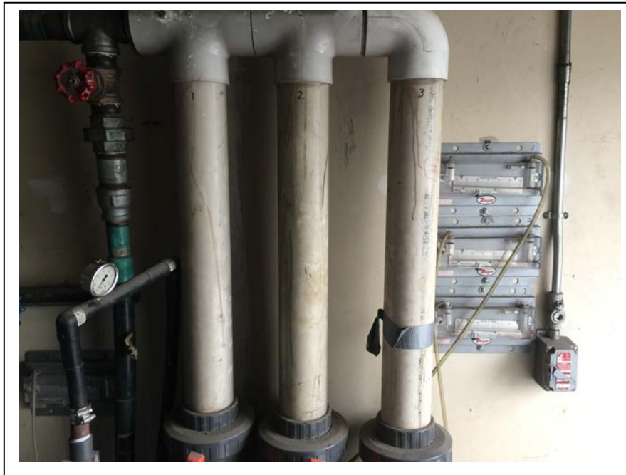
Photo 2: Looking at the VES lines of the remediation system. (July 10, 2018)
