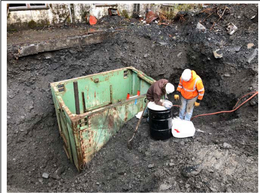
Photo 7: Looking northwest at the trench box placed in excavation to access and inert the tank. (October 4, 2017)
