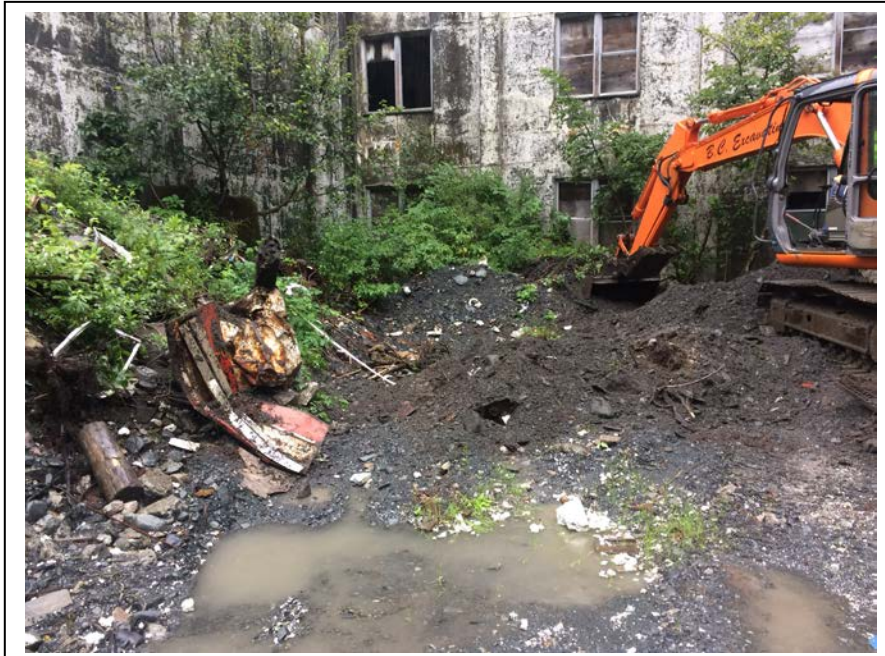
Photo 3: Moving stockpiled soil overlying the UST. Vehicle and building debris were present in the soil. (August 29, 2017)
