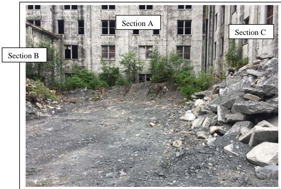
Photo 2: Looking northwest at the location of the UST, prior to removal. (July 6, 2017)
