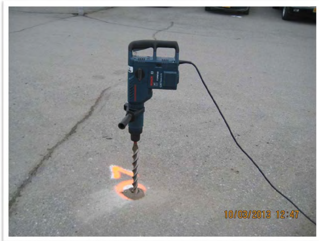
Photograph 1 – Drilling a hole in soil at location M-07 (3/4-inch-diameter by 32-inch drill bit). View to the east.
