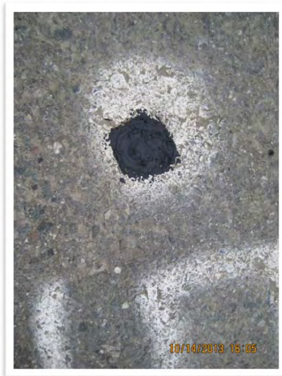
Photograph 10 – Cold patch was installed in the top 4 inches, then holes were sealed with elastic crack filler.
