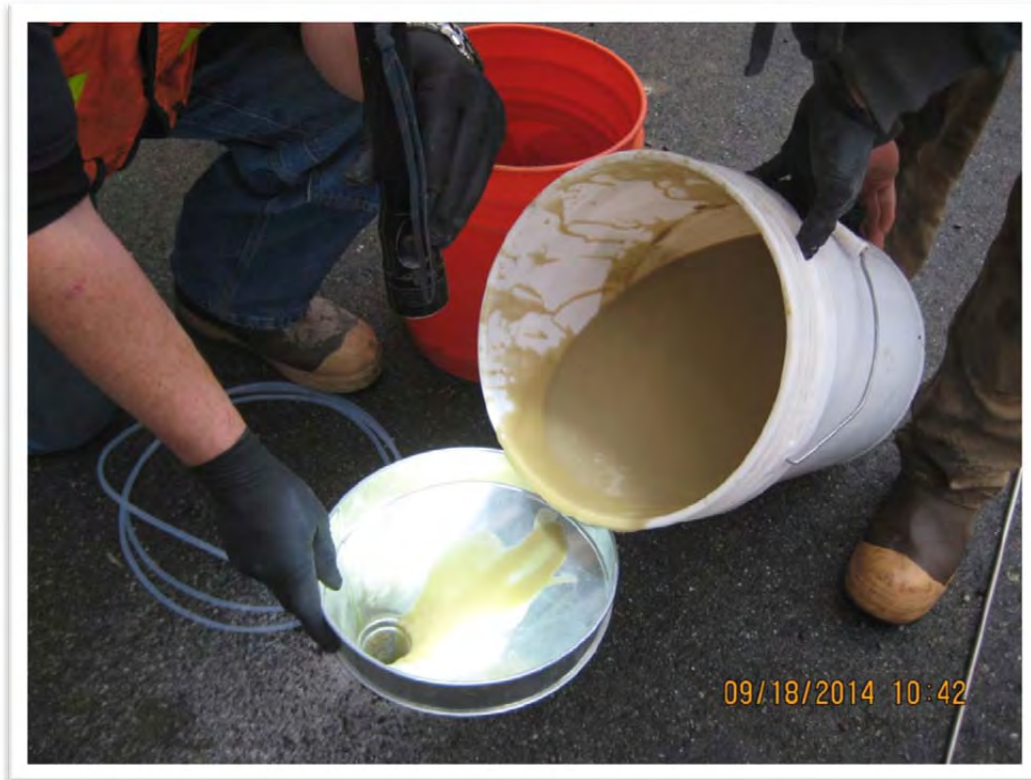
Photograph 5 – A grout slurry was added above the sand pack to seal each soil gas monitoring well.
