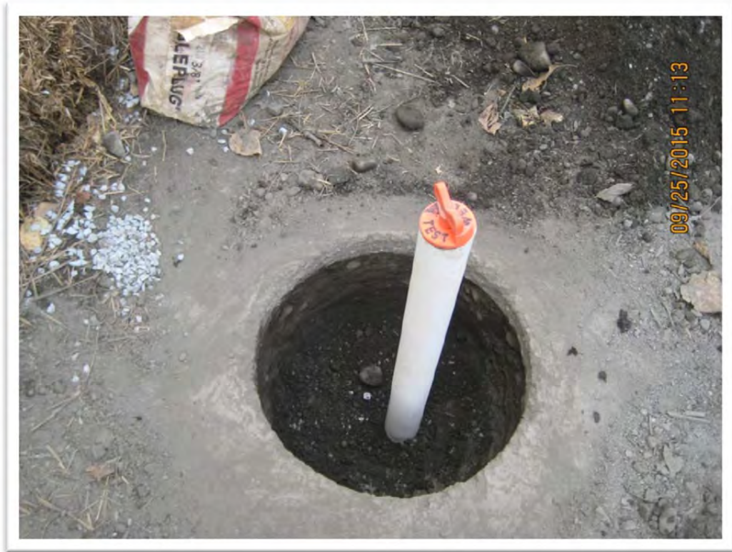
Photograph 3 – Soil borings were completed as 2-inch-diameter wells; sand was placed around pre-packed well screens, and the wells were then sealed with hydrated bentonite chips.
