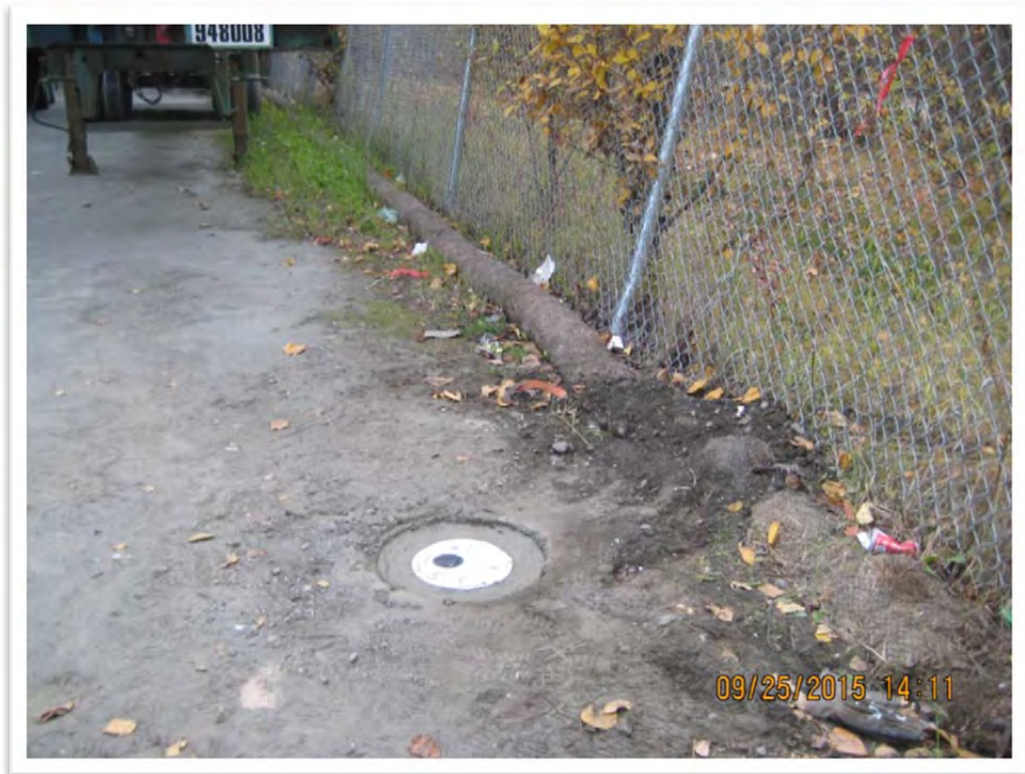
Photograph 4 – Photograph of well MW-7 with flush mount completion in concrete. View to west.
