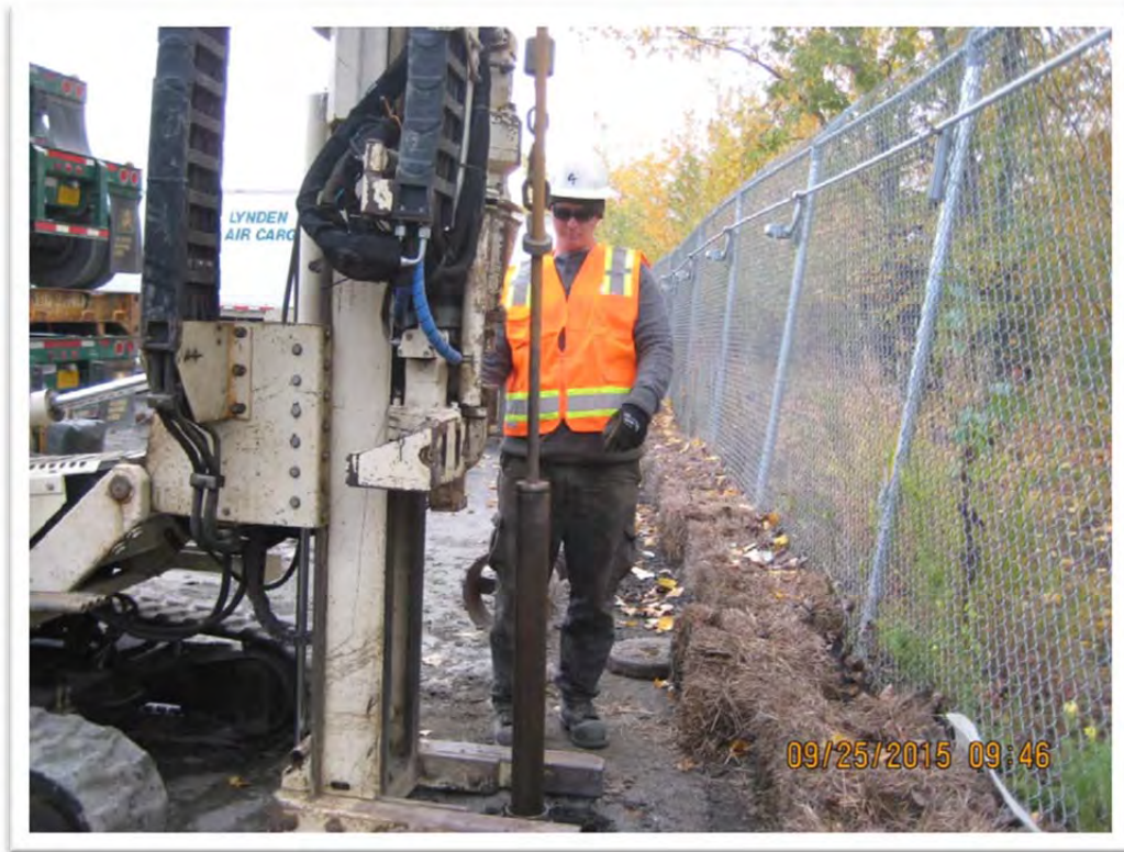
Photograph 1 – Removing soil core from SB-1/MW-6. Soil borings were installed using a Geoprobe 6610 drill rig. View to Northeast.
