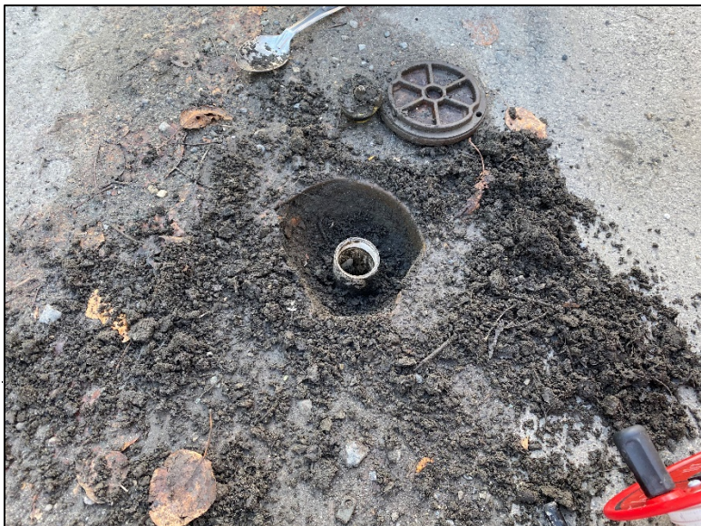
Monitoring well CHMWE5; not sampled
