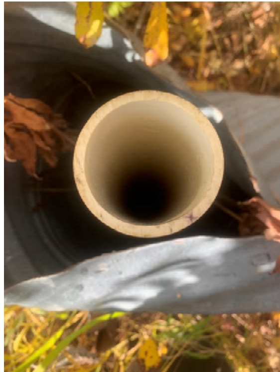
FG-15 overhead shot – note crushed protective culvert, well undamaged
