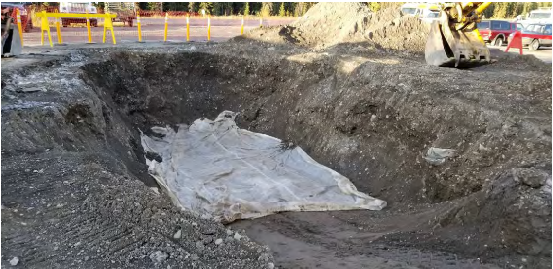
Photo 6: September 17, 2019, looking north - This photo shows the plastic barrier that was placed in the excavation prior to backfilling with the soils from the presumed clean stockpile.
