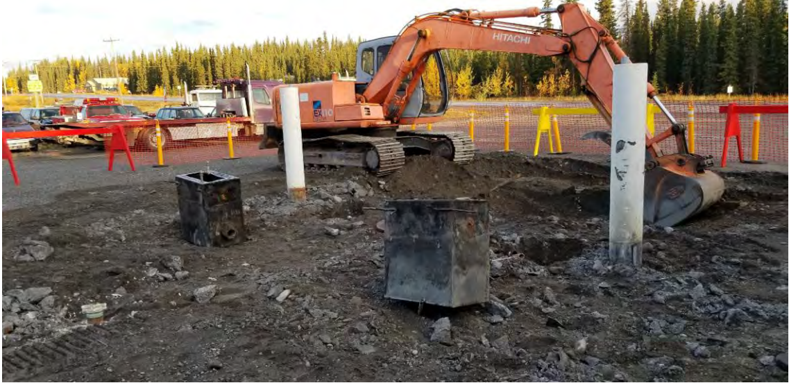
Photo 3: September 17, 2019, looking northwest – This photo shows removal of the dispenser boxes following the removal of the apron and island.
