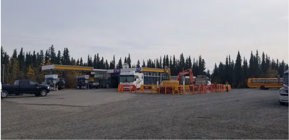
Photo 1: September 16, 2019, looking southeast - This photo shows the Glennallen Fuel and Service gas station. The UST is located within the barrier fence.
