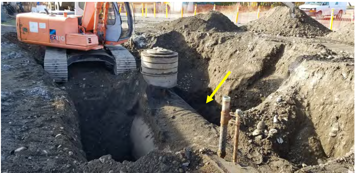
Photo 4: September 17, 2019, looking south - This photo shows the excavation of the tank in the area of the sump. There was evidence of a release from the sump and soils in the area right (west) of the sump (arrow) were impacted.
