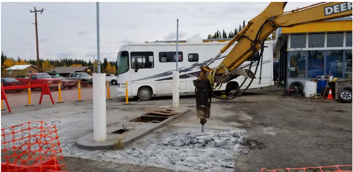
Photo 2: September 16, 2019, looking east - This photo shows the dispenser island and concrete apron. The dispensers were removed sometime in the past, but the vent lines and island remained.
