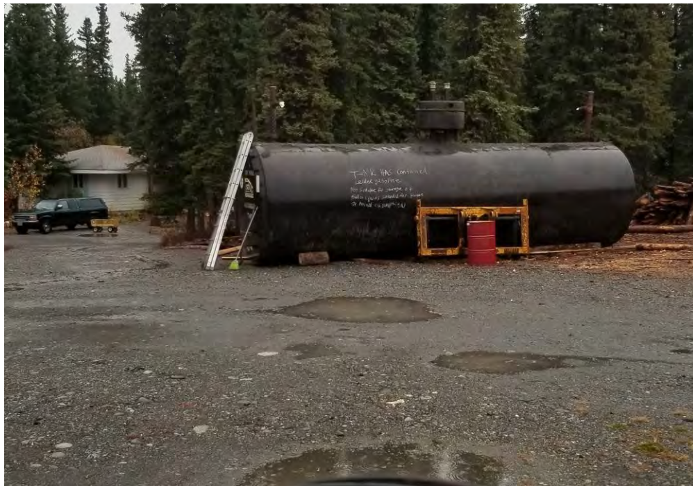
Photo 8: September 19, 2019, looking southeast - This photo shows the tank following removal. The tank was rinsed and collected water transported for disposal. The tank was sold to a private party.
