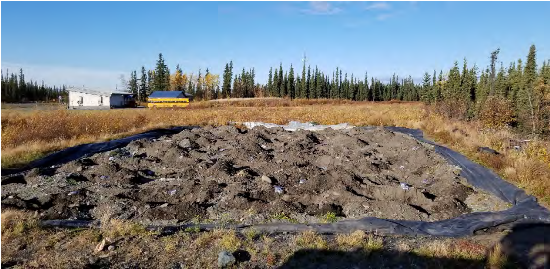
Photo 2 (9/19/2019 – looking west): This photo shows the landfarm during the sampling event after all test pits have been excavated. The sampling event results in significant mixing of soils which may be considered as a mixing/till event.
