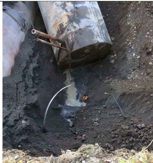
Photo 9 Groundwater seeping in under UST #3 as it is pulled out of the excavation pit. (10/10/17)
