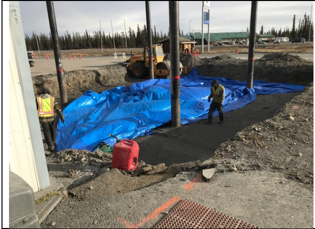
Photo 13 Looking Northeast. Plastic tarp being placed as a visible indicator of the top of the clean fill brought in from off site. (10/24/17)
