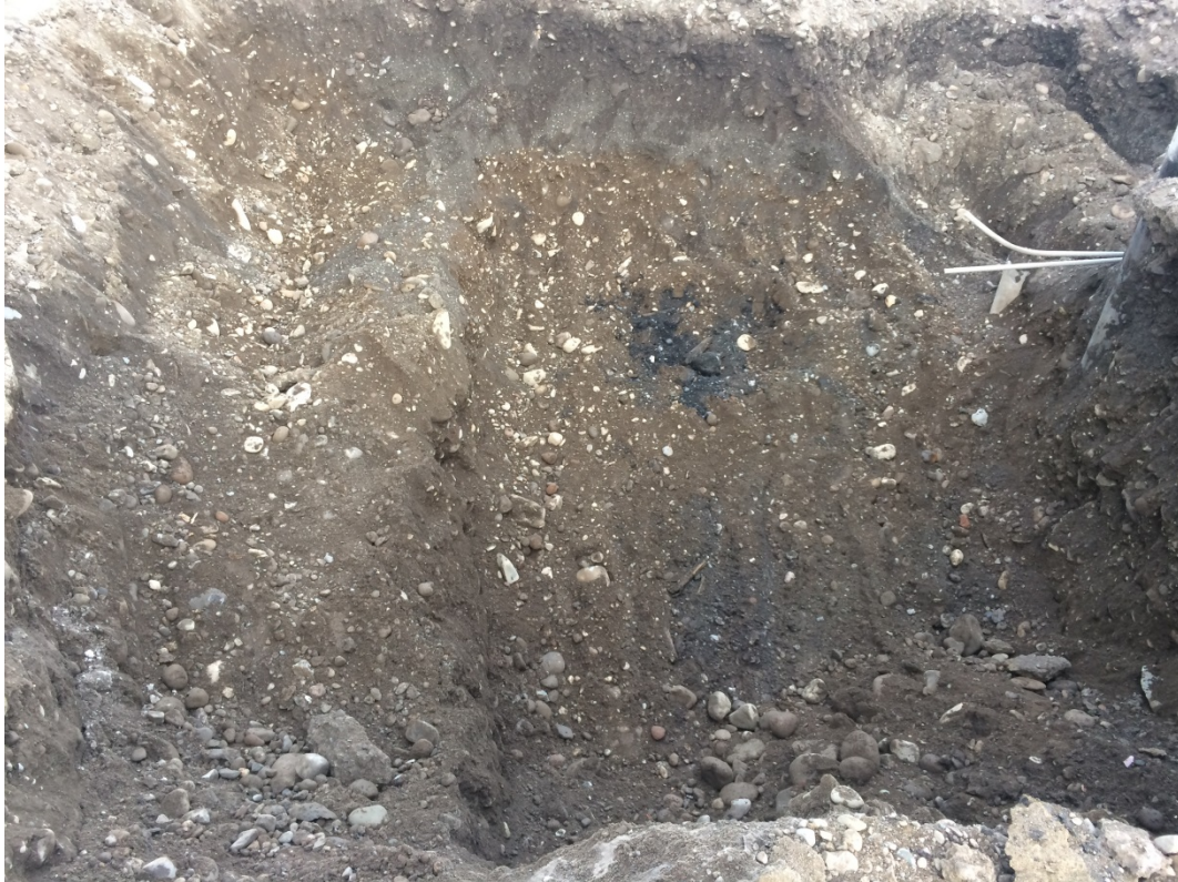
Photo 1: Burned debris encountered during excavation of the release from the first fuel island. Looking Northwest (10/21/2017)
