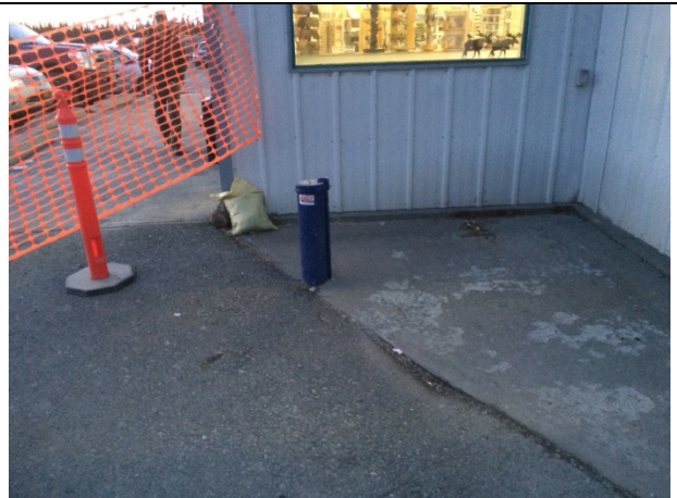
Photo 10 Non-Potable water well . Looking West (10/22/17)
