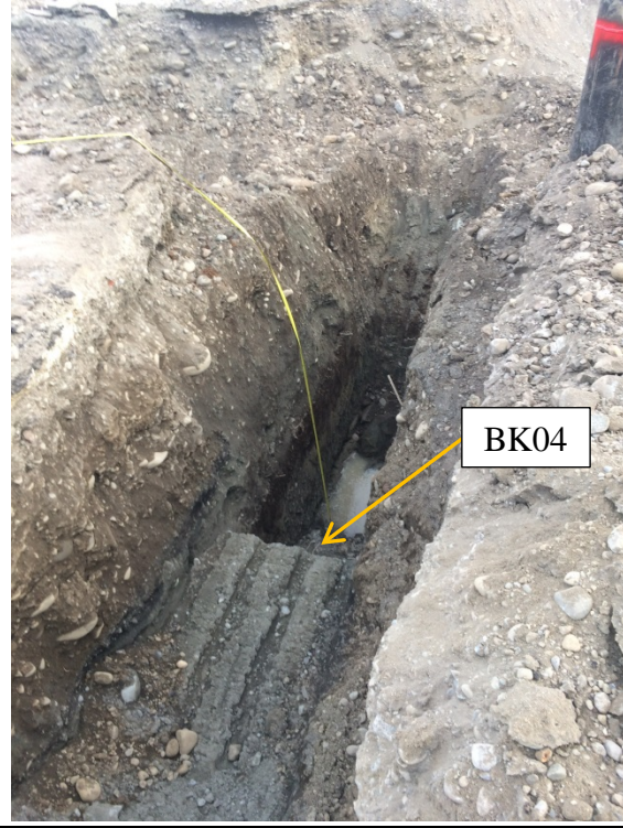
Photo 4 Deep test pit dug at the release site from the middle fuel island. Looking East (10/21/17)
