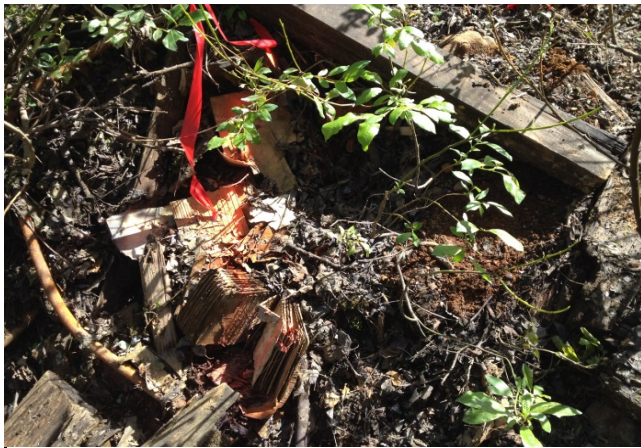
Photo 3. Open pit, broken battery plates prior to being placed in drums. 7/1/2014
