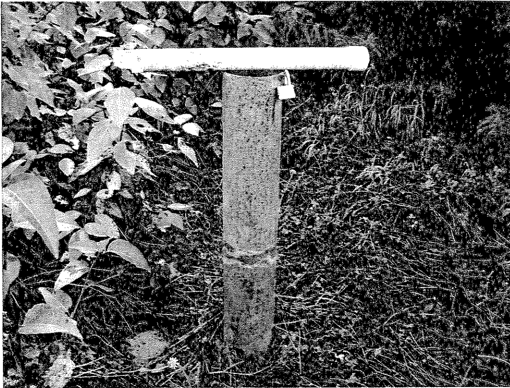
Photograph 1: GW-1 with broken casing piece.
