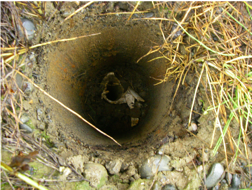
Photograph 2: Broken casing in ground, GW-1.
