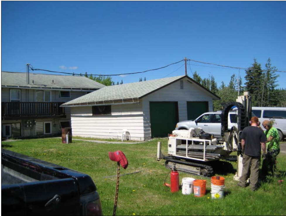
Photo 03 - Looking northwest at installation of SB-02; SB-01 location near drum in background
