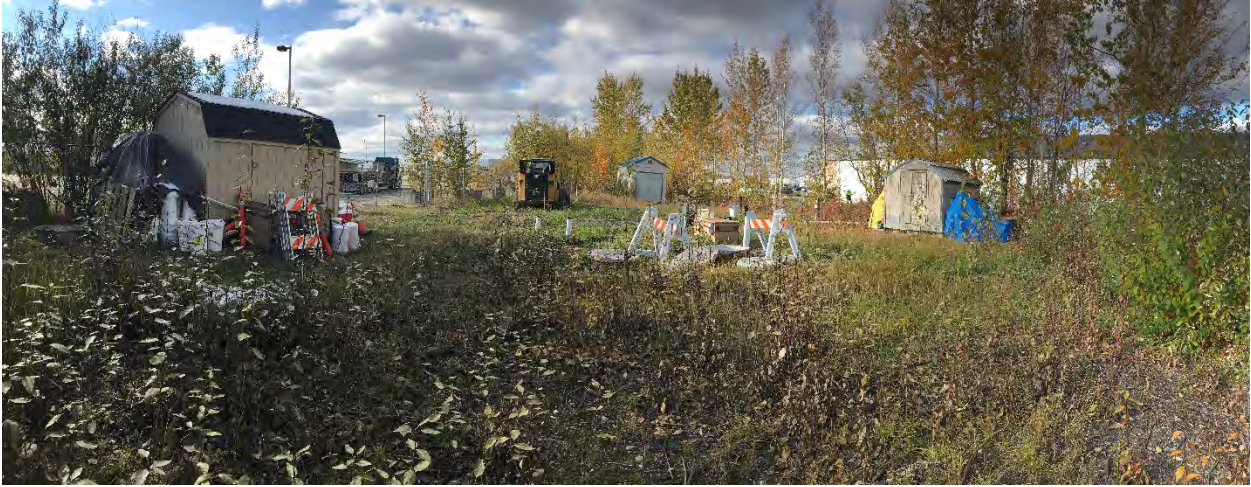
Photo #1 – Panoramic View of Site Prior to Start of 2021 Drainfield Installation (looking west)
