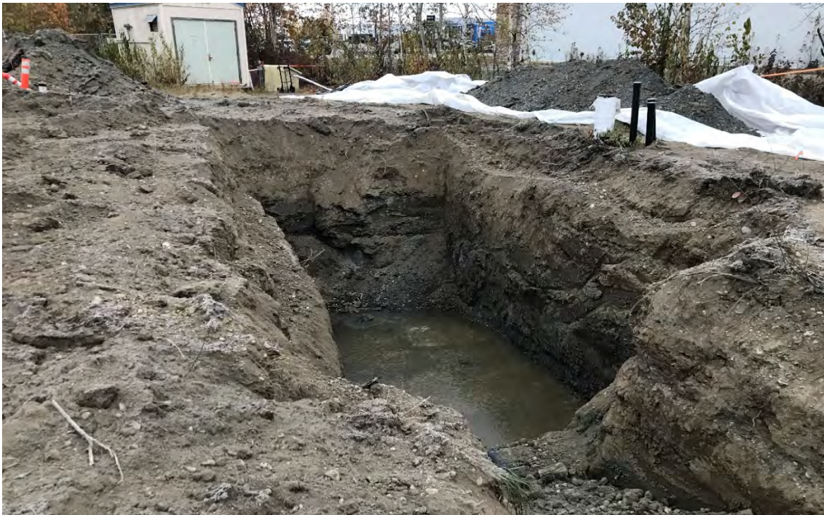
Photo #4 – Excavation of Trench (looking west) towards Shed for WRW well. Note dark stained soil strata at bottom of trench. Note the stockpile of contaminated soil in the background.
