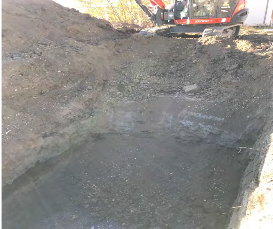
Photo #3 – Excavation of West End of Trench. Note stained soil strata near bottom of excavation.
