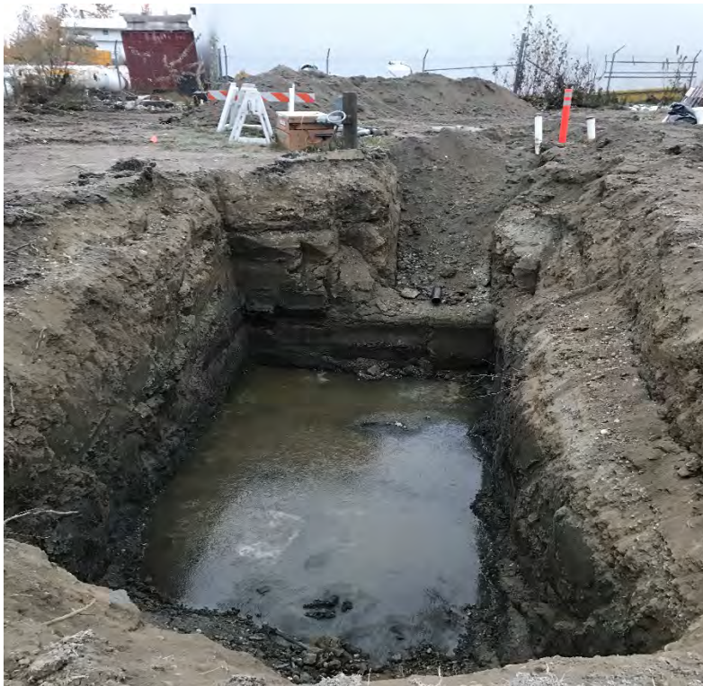
Photo #2 – Start of East End of Trench Excavation (looking east). Note sheen on groundwater and stained contaminated soil strata at bottom of trench.
