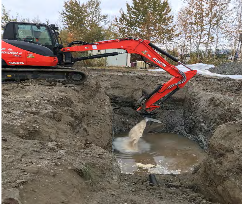
Photo #5 – Application of Klozur™ CR powder on the bottom of trench in contaminated groundwater.
