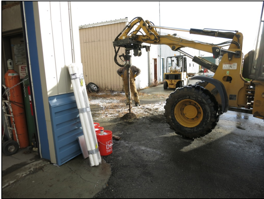
Photograph 3: Photo shows auger mounted on loader drilling MW-3R. Southeast corner of Alaska Airlines terminal building is visible on the left. (Sep 30, 2015).
