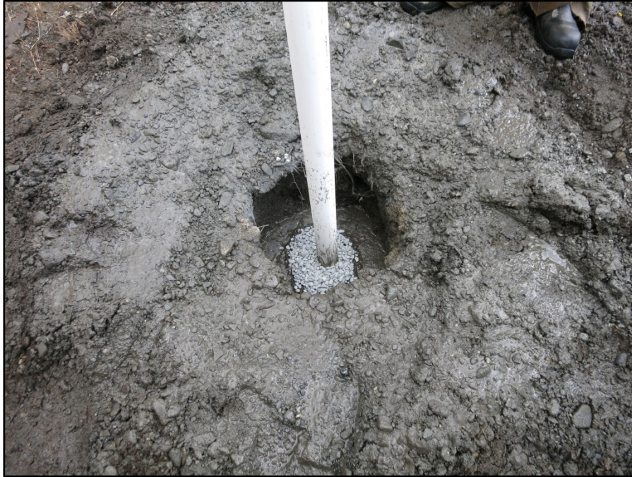
Photograph 5: Installing monitoring well in boring MW-3R. Bentonite well seal is visible. (Sep 30, 2015).
