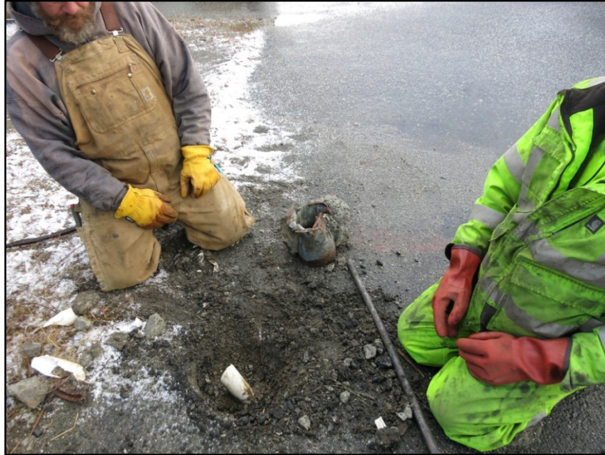
Photograph 1: Damaged and unreparable well MW-3, about to be decommissioned. Mangled surface vault has been removed and is visible at photo center. (Sep 30, 2015).
