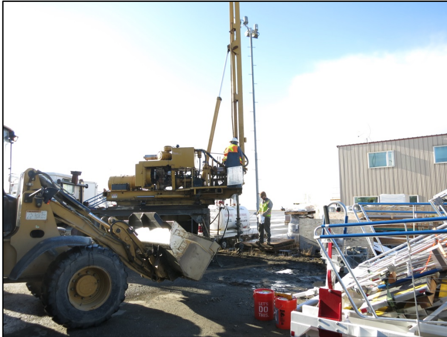
Photograph 6: Large truck-mounted auger drill rig drilling MW-1R. Photo faces southwest, away from Alaska Airlines terminal building. (Sep 30, 2015).
