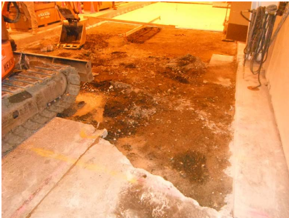
Photo 2: Excavation Area A – Exposed area with fuel hydrocarbon odor.
