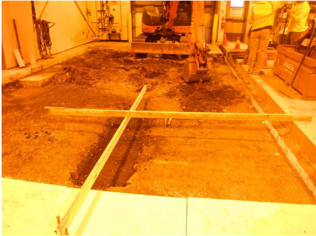
Photo 1: Excavation Area A – Exposed area with fuel hydrocarbon odor.
