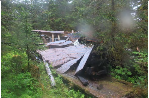
Photo showing a collapsed building that TPEC believes was an old pulley house.
