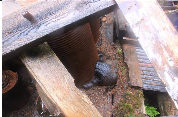
Drums containing solidified Bunker C. Drums were within the wreckage of the collapsed pulley house.
