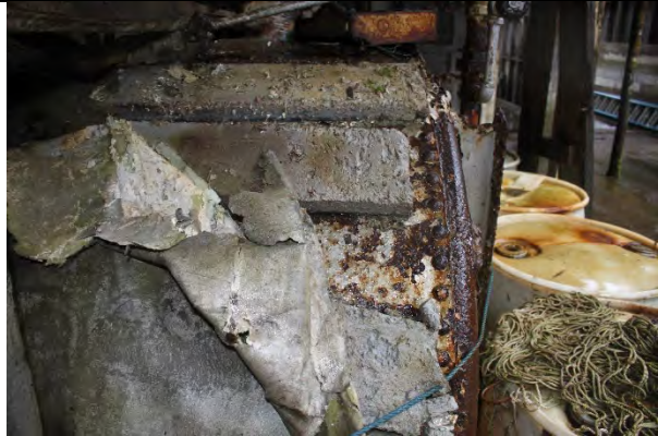
Photo showing insulation on boiler located on dock that may contain asbestos.
