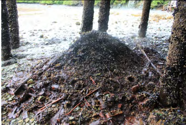
Bunker C mixed in with pile of metallic debris. Pile was below a hole in the floor located in the shop above.
