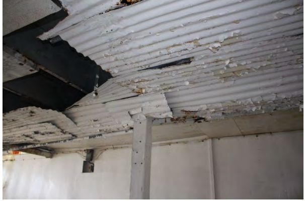
Photo showing peeling paint chips within Meat/Shop Building on Dock. Paint chips may contain lead.
