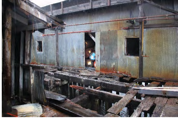
Photo looking into a door on the Boat Building. Several 55-gallon drums were observed.
